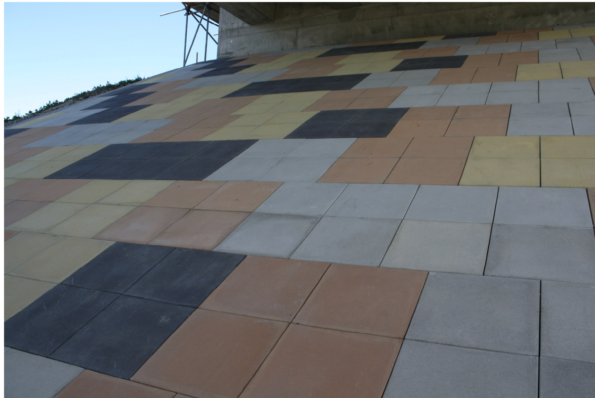
Coloured concrete panels on CSM1 abutment to represent an aerial view of the Canterbury Plains
