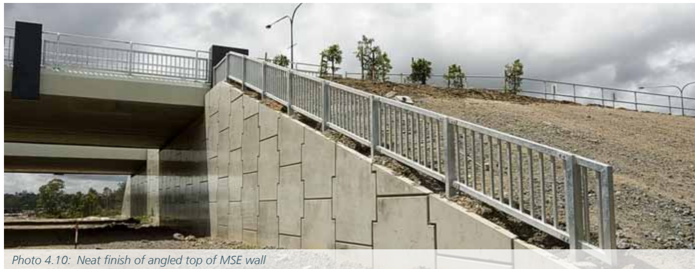
Photo 4.9: Vertical MSE retaining wall wrapped around bridge abutment
