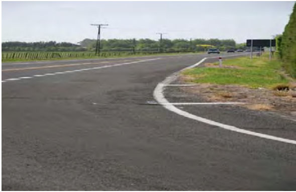
Photo 5: Patchwork repair zone located on corner. Source: Yvonne Forrest (MOTO)
