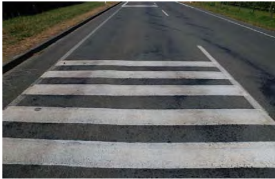
Photo 7: Transverse road markings located across the lane in break zone.
