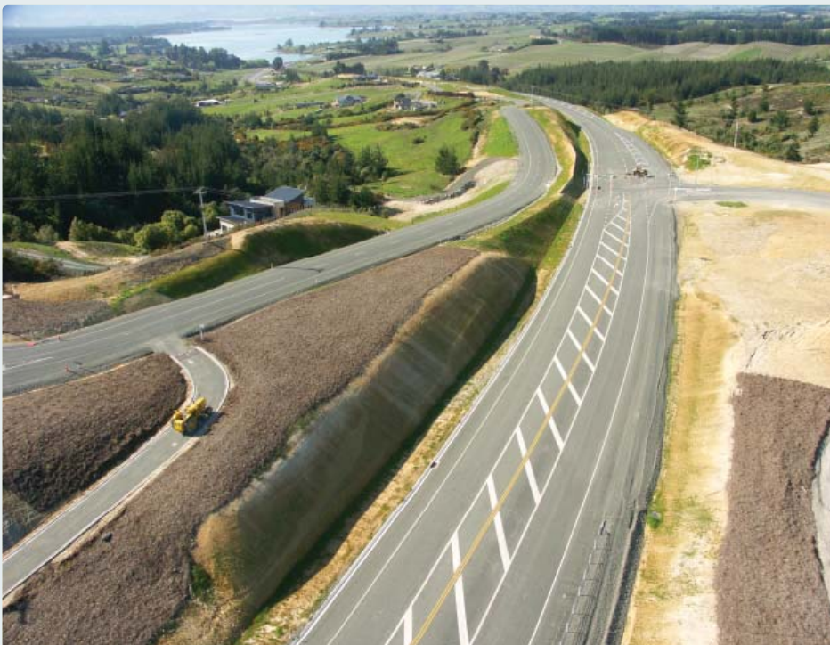
The chipseal is down, the line markings are laid and the new highway is finished and ready for traffic.
