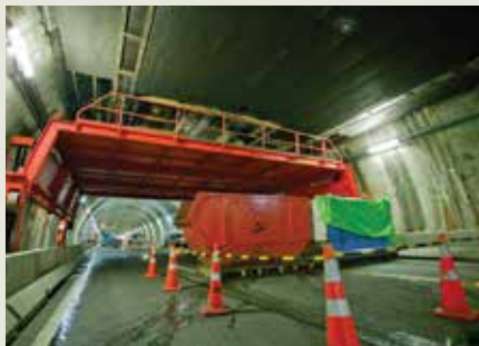
THE 'THUNDERBIRD 7' - MUCH OF THE WORK ON THE TUNNEL TOOK PLACE AT NIGHT, AND THE THUNDERBIRD 7 PROVIDED A SAFE AND STABLE PLATFORM FOR WORKERS DURING THE DEMOLITION OF THE OLD CEILING. BECAUSE THE PLATFORM COULD REMAIN IN THE TUNNEL THROUGHOUT THE UPGRADE, LONGER SHIFTS COULD BE WORKED EACH NIGHT AND STILL HAVE THE TUNNEL READY TO OPEN EACH MORNING.
