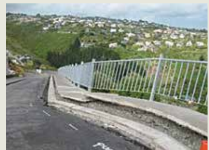
DAMAGE FROM THE FEBRUARY 2011 EARTHQUAKE - ROTATED GABION BASKET RETAINING WALL, GLENSTRAE ROAD, REDCLIFFS, CHRISTCHURCH.
