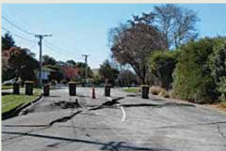
LATERAL SPREADING FROM THE SEPTEMBER 2010 EARTHQUAKE - LOCKSLEY AVENUE, DALLINGTON, CHRISTCHURCH.
