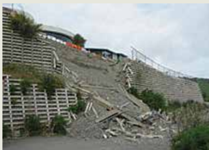
DAMAGE FROM THE FEBRUARY 2011 EARTHQUAKE - COLLAPSED CRIB WALL IN GALILEE LANE, SUMNER, CHRISTCHURCH.
