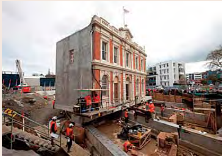
⌘ MOVING THE ROB ROY HOTEL AS PART OF THE VICTORIA PARK TUNNEL PROJECT.
