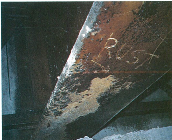
Figure 4.4: Failure of wax barrier coat.
