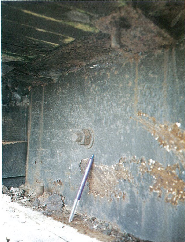
Figure 4.3: Coating failure caused by inadequate primer.
