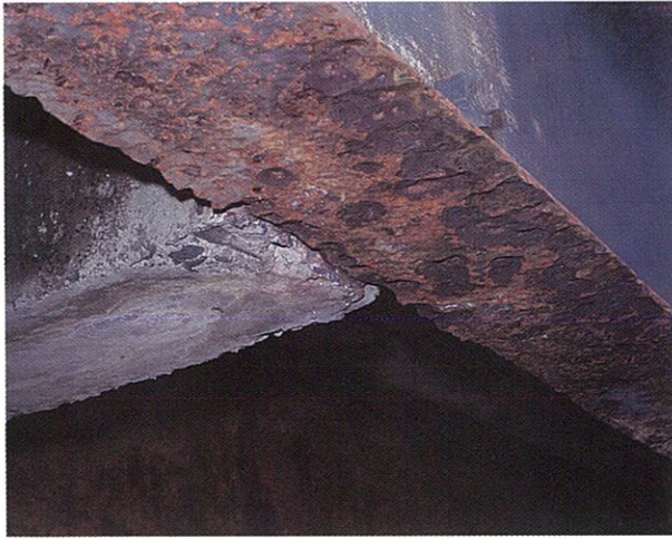
Figure 4.9: Loss of section: severe pitting due to condensation and concentration of salts on bottom flange (and lack of maintenance).
