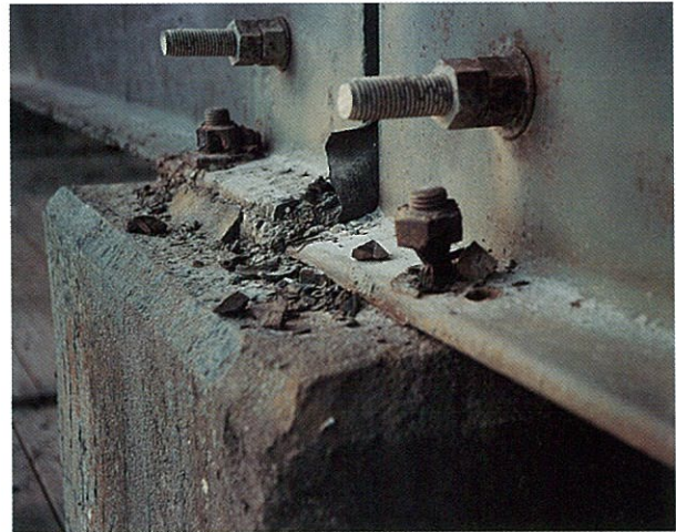
Figure 4.10: Debris around bearings retains moisture.
