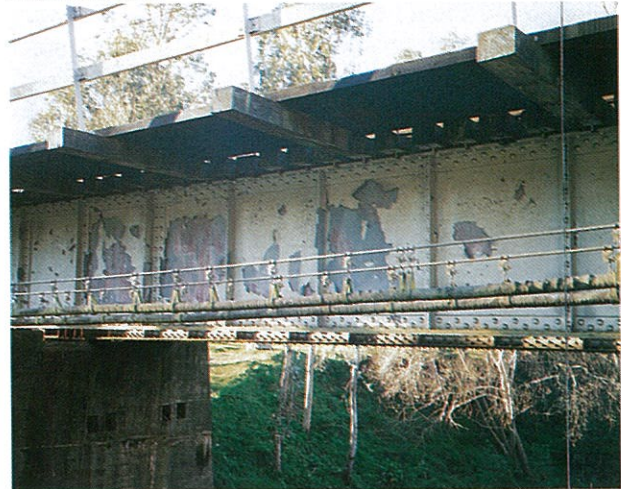
Figure 4.5: Incompatible coatings (alkyd paint over zinc-rich).
