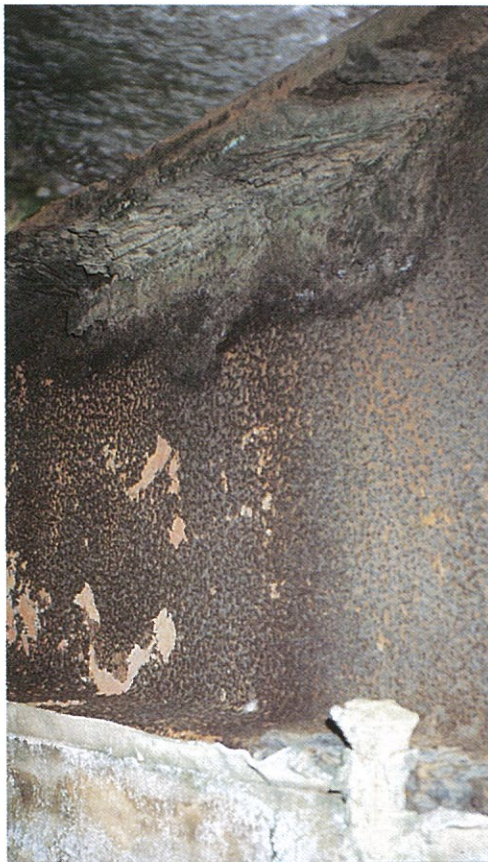
Figure 4.7: Damp patch caused by accumulated rust and debris.
