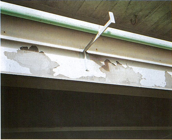
Figure 4.6: Loss of adhesion (inadequate surface preparation).
