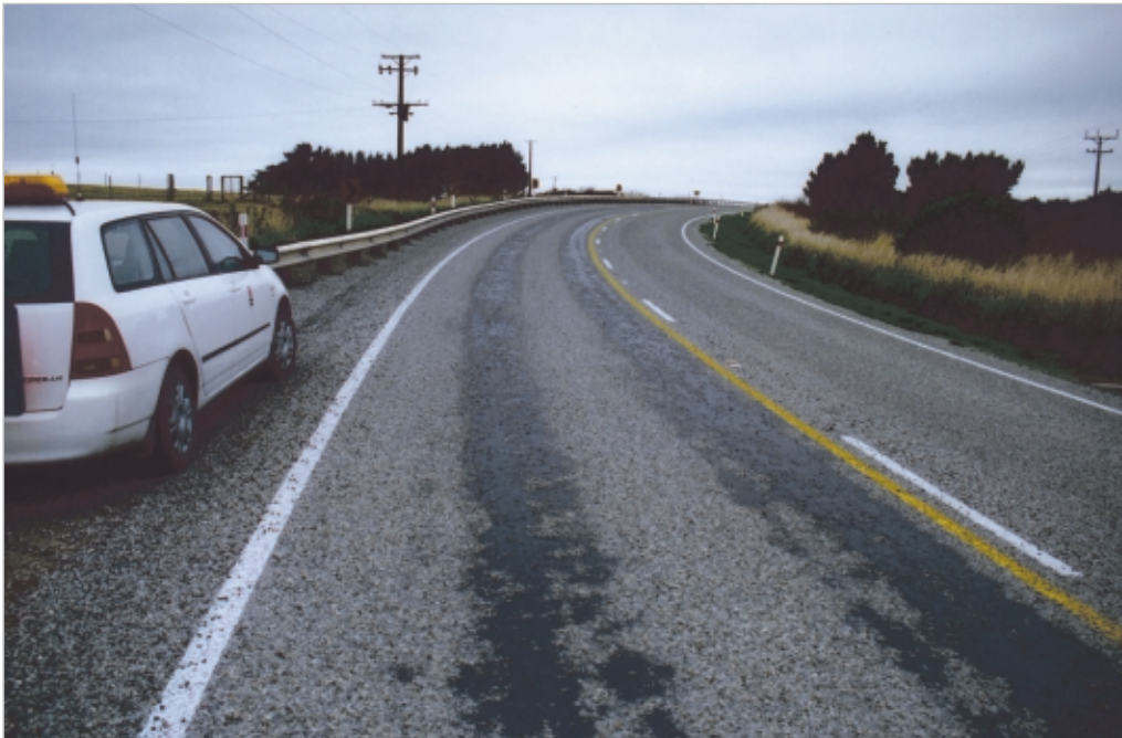
Figure 12-5 Chip loss can occur within 48 hours after chipsealing. Photo courtesy of Les McKenzie, Opus
