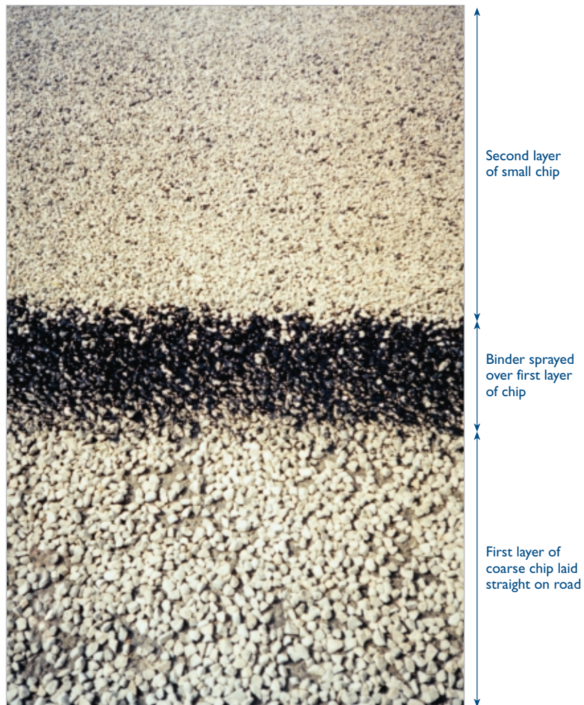
Figure 12-8 The three layers of a sandwich seal are shown part way through construction.
