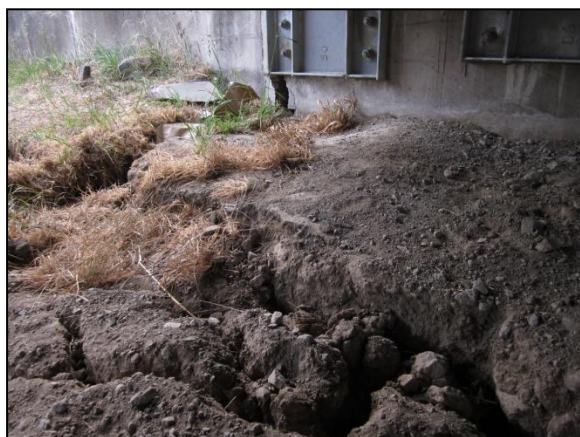
Figure HO3 Cracking from down-slope movement at abutment at Lyttelton end.
