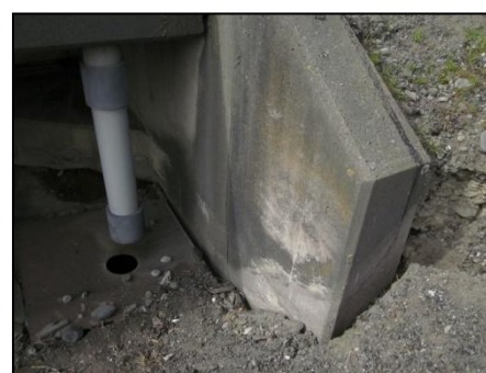
Figure C6 Settlement at abutment.
