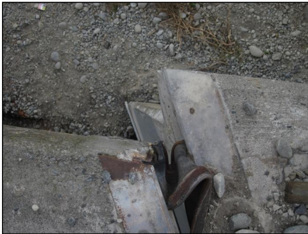
Figure BS8 Horizontal rotation at south-west corner.
