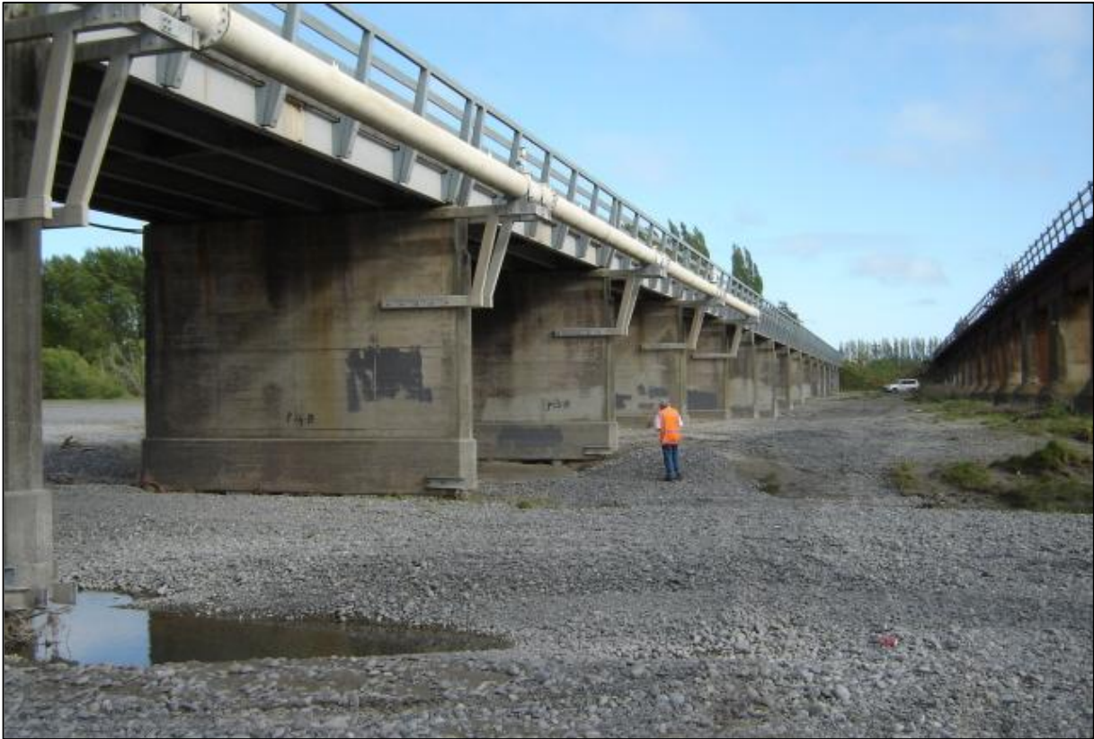
Waimakariri River (Main North Road) Bridge, looking north. (Railway bridge on the right)
