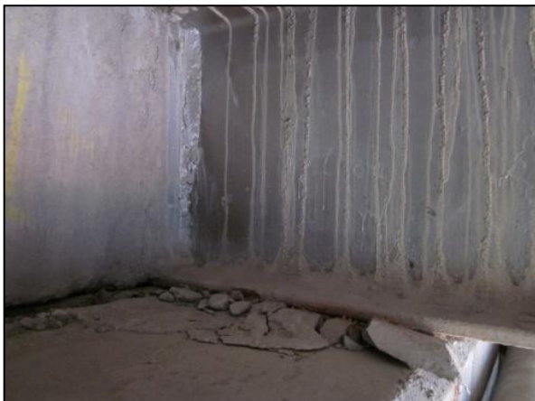
Figure W2 Damaged mortar seating under beam at south abutment.
