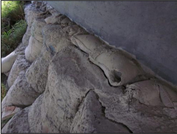
Figure W4 Cracked underpinning at south abutment.
