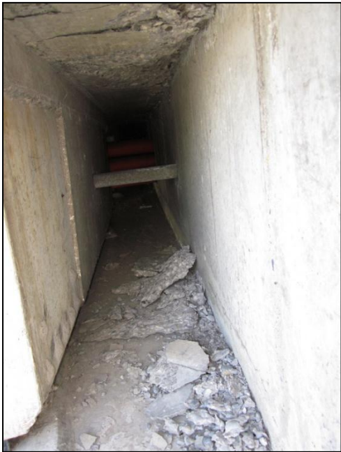
Figure R2 Pounding damage at north abutment.
