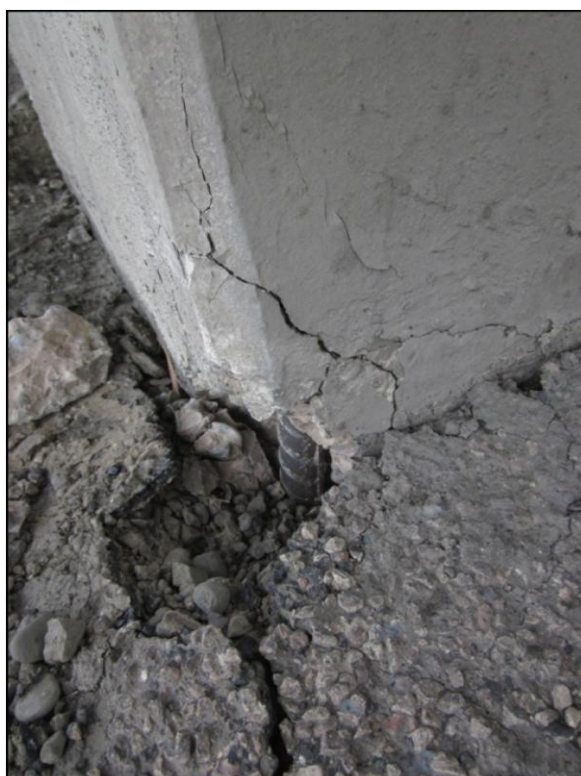
Figure PH1 Spalled concrete and buckled column reinforcement.
