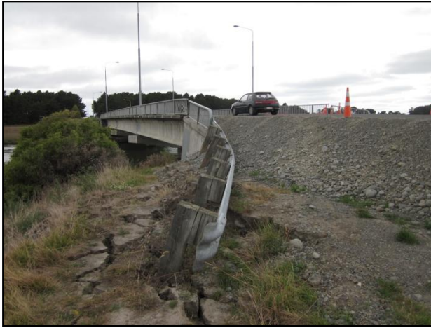
Figure BS6 Lateral spreading on west approach.
