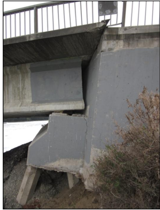
Figure BS7 Settlement and rotation at west abutment.
