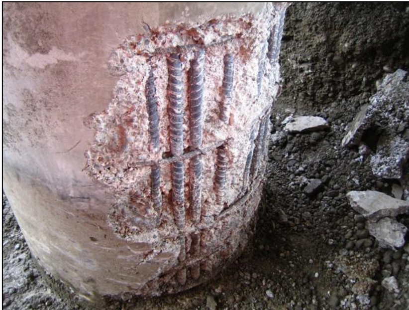
Figure O1 Spalling damage at the base of the south column of the eastern pier. The cracked concrete has been removed to reveal poorly compacted concrete around some of the reinforcing.
