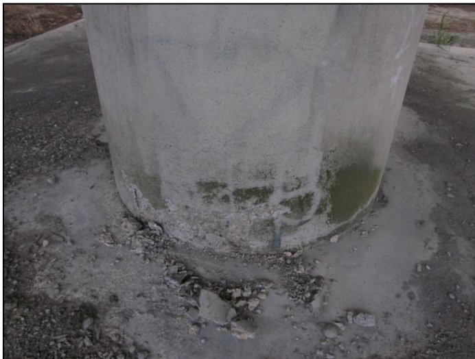
Figure ST1 Spalling in pier of Bridge No 2.
