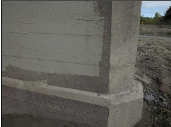
Figure W6 Horizontal crack in Pier 23 400 mm above pilecap.
