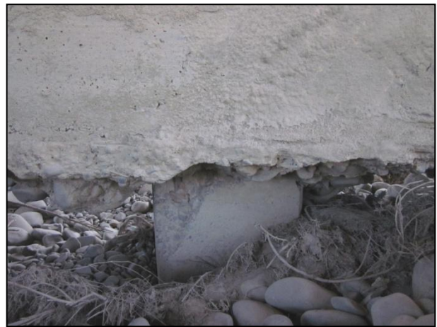
Figure HA2 Spalling in pile under pier pilecap, probably due to transverse loading on bridge.
