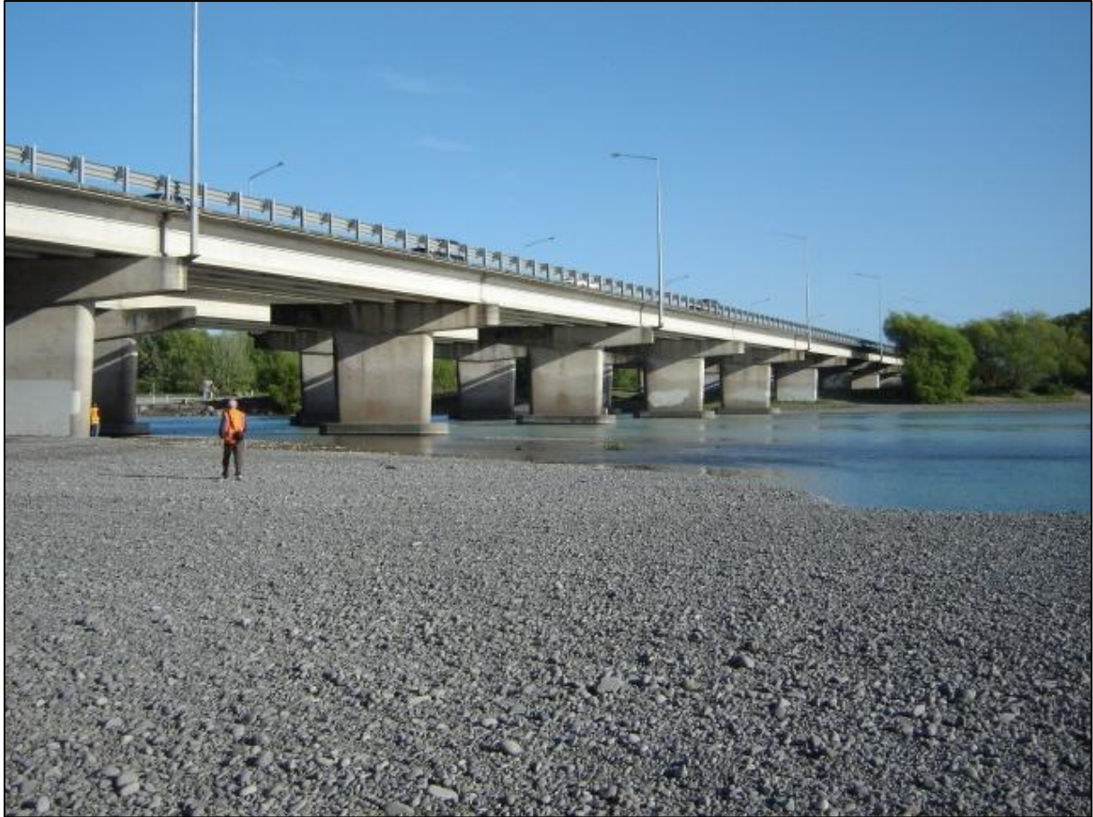
SH1 Waimakariri River Bridge (southbound and northbound). Central six spans of seventeen, looking north-west.
