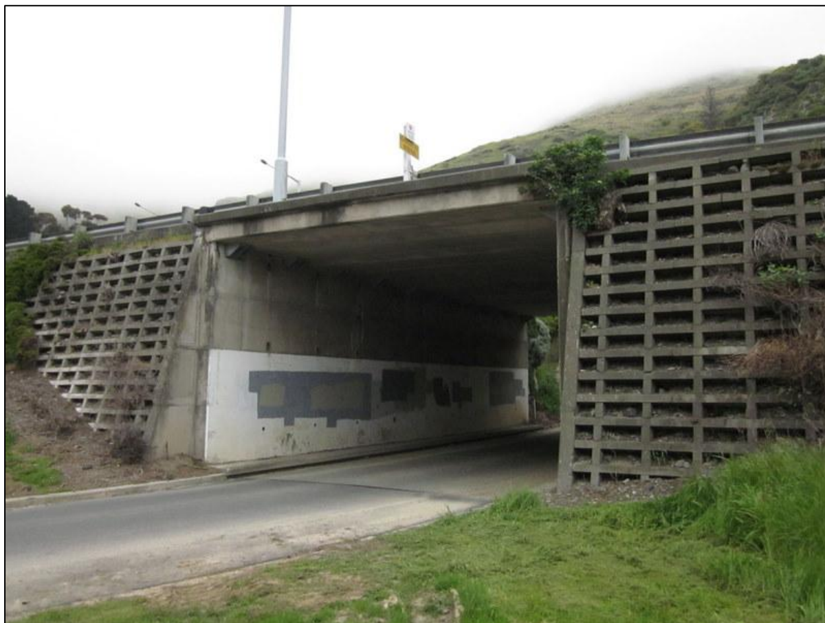
SH74 Heathcote Valley Overpass, looking south. (Note retrofitted anchor brackets at top of wall.)
