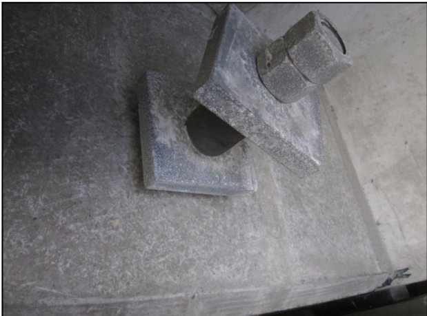
Figure R4 Loose linkage bolts at south abutment.
