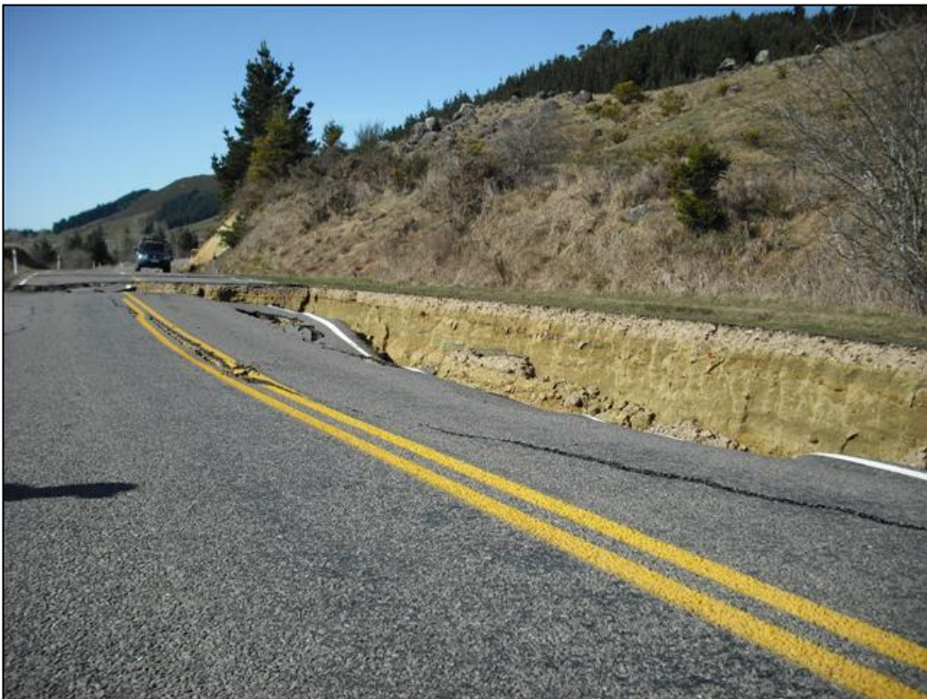
Figure 9. Earthquake induced landslide affecting road (SH77)
