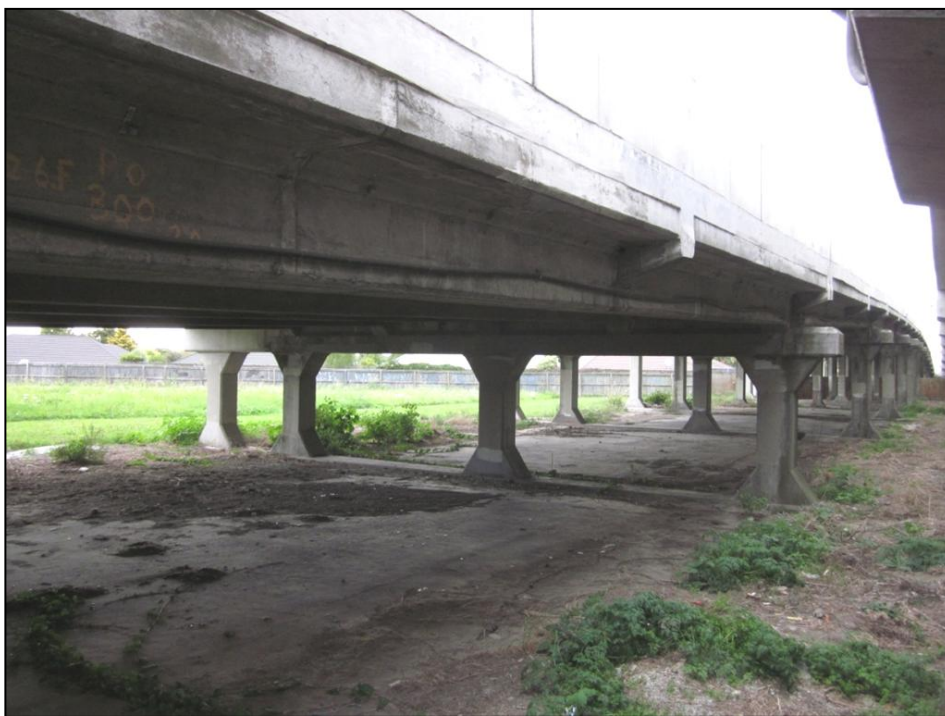
Bridge No 1 (Southbound), looking South; built in 1937. Central spans of fifteen total. Note extension on far side, added in 2006.
