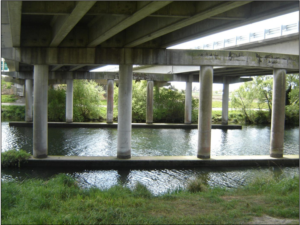
SH1 Kaiapoi Railway and River Bridge, looking north, (span three of six).
