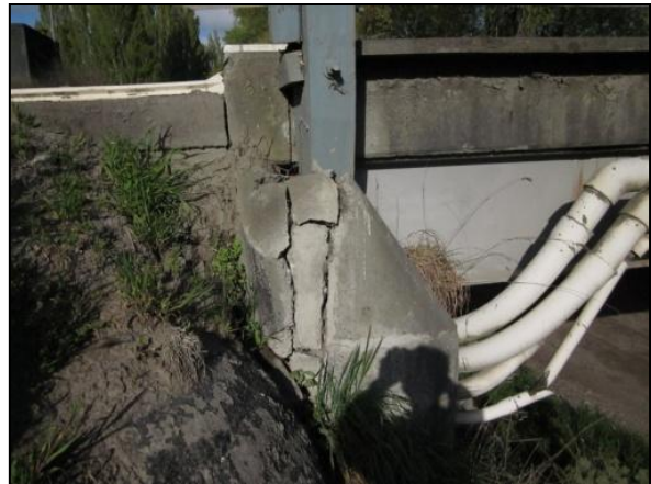
Figure W1 Damaged abutment return wall at south abutment.
