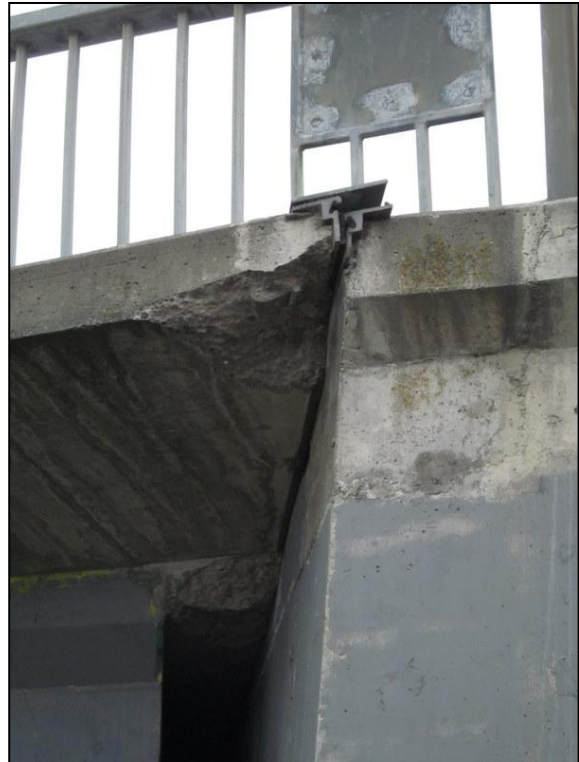
Figure BS2 Joint closed at north-west corner.
