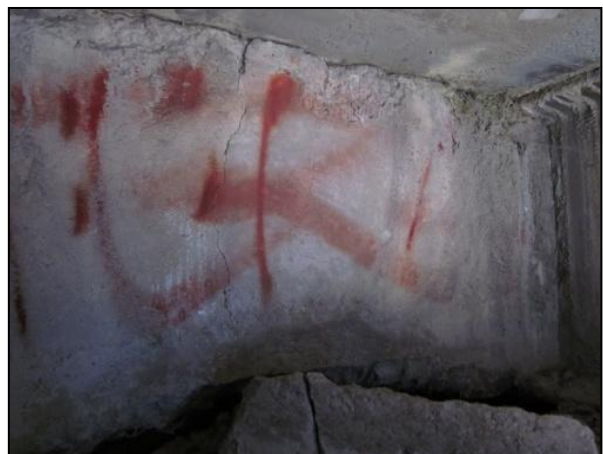
Figure W3 Cracked and spalled diaphragm at south abutment.
