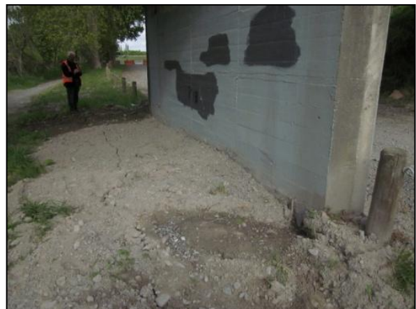
Figure W7 Cracking in ground around Pier 29.
