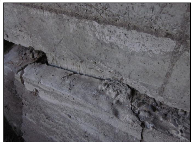
Figure HA4 Cracking indicating possible longitudinal displacement.
