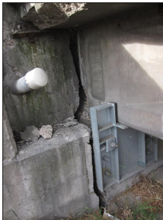
Figure HO4 Cracking in abutment at Lyttelton end.
