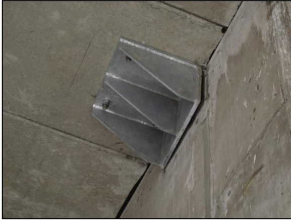
Figure HVO1 Shear bracket on underside of deck units.
