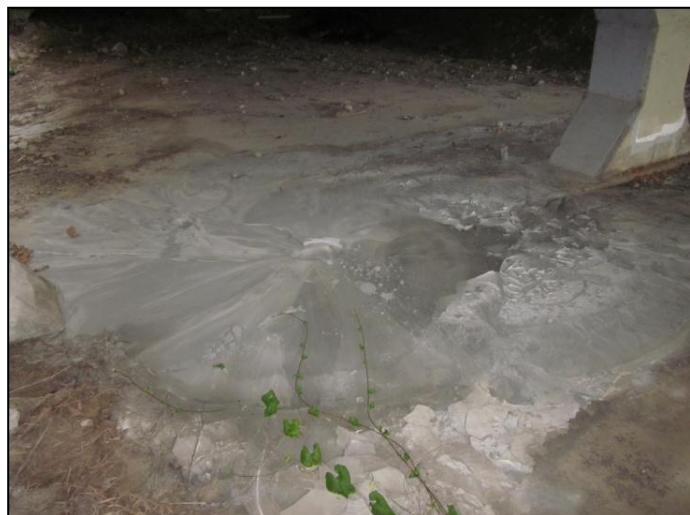
Figure ST2 Sand boils near Bridge No 1 pier.
