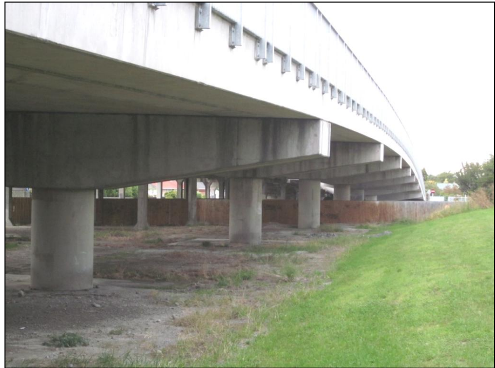
Bridge No 2 (Northbound), looking South; built in 2006. Central spans of nine total.
