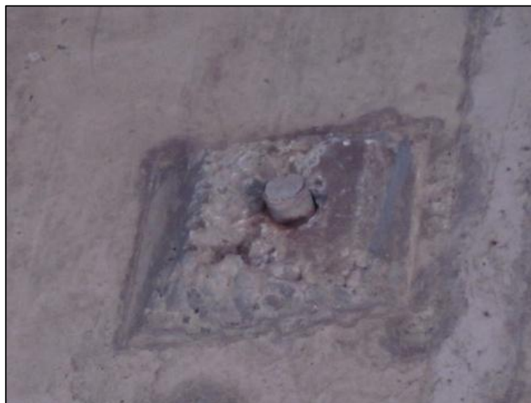
Figure K2 Fractured linkage bolt in pier diaphragm.
