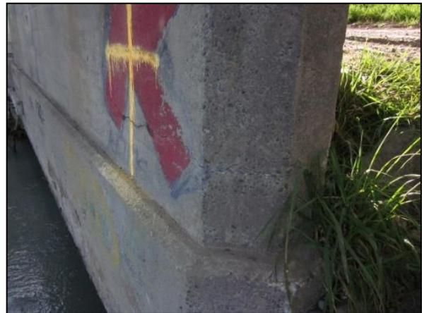
Figure W5 Horizontal crack in Pier 2.
