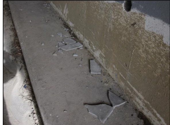
Figure HVO2 Mortar on ground from brackets above.
