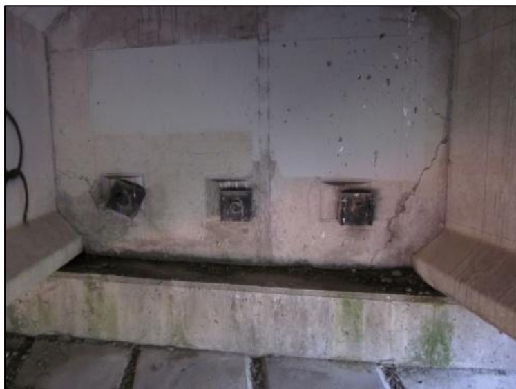
Figure K1 Damaged diaphragm at abutment.
