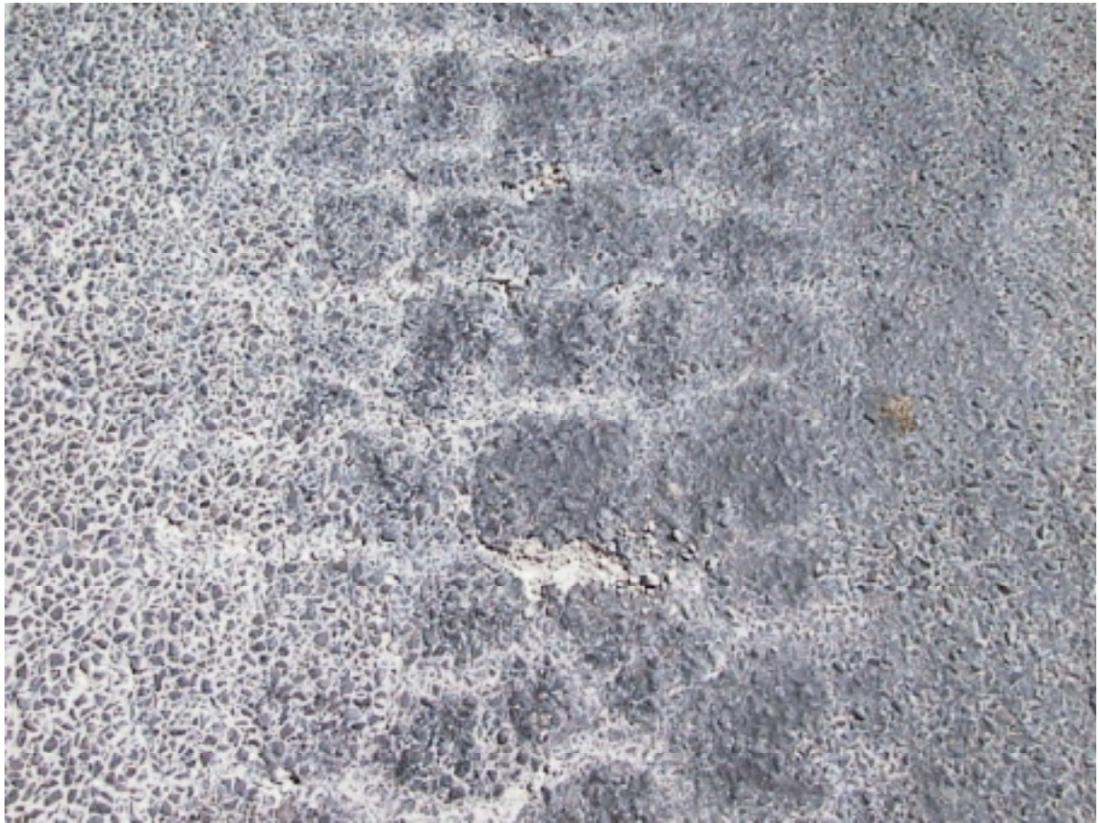
Figure 8.4 Onset of erosion at the crack edges.
