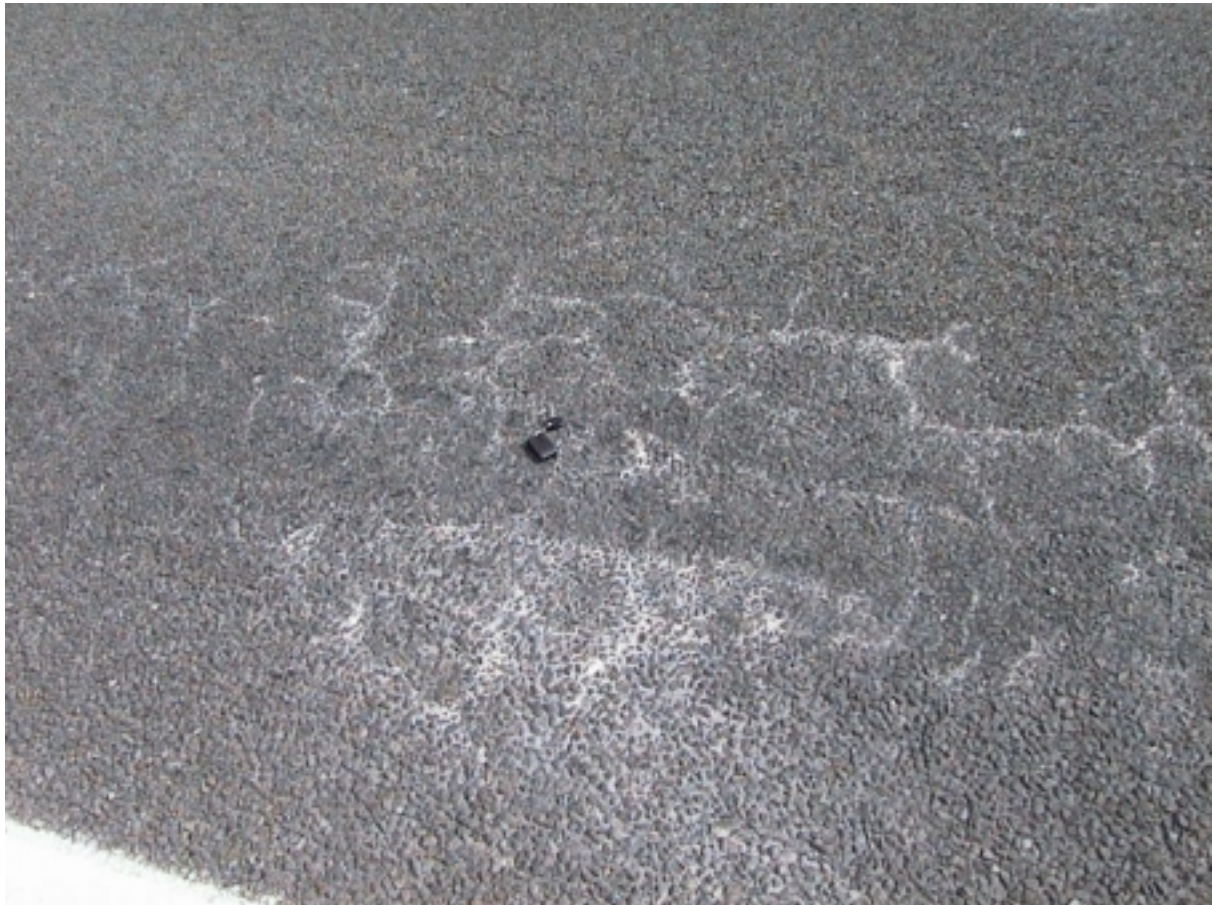
Figure 8.3 Onset of fatigue cracking reflecting through the surface.
