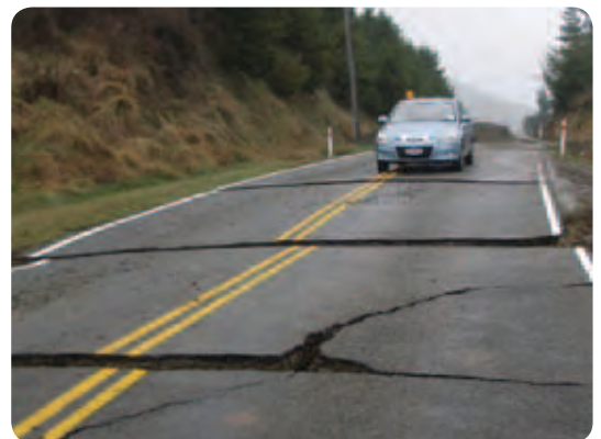
February quake damage at Glenroy, State Highway 77, Canterbury - between Windwhistle and Glentunnel
