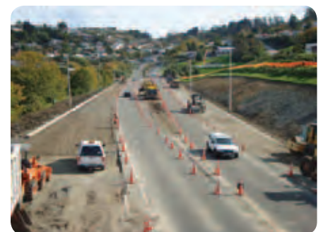
Work on four-laning the Goodall Street pedestrian bridge to Barnes Drive section of the Caversham Highway Improvements project
