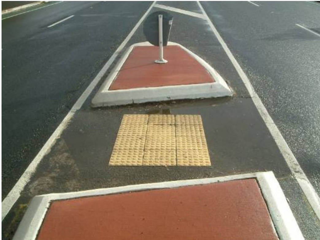
Photo 10: Warning indicators correctly installed across the full depth of this pedestrian median island (1.2 - 1.8m deep). Note: Warning indicators should cover full width of cut through. This one could be bypassed.
