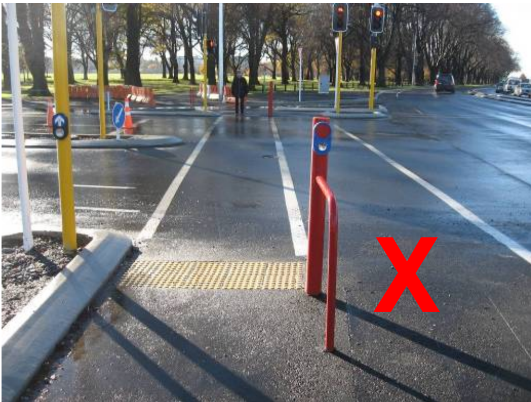
Photo 22: The TGSI at this signalised pedestrian and cyclist crossing are installed across the pedestrian area only. The TGSI should extend across the entire facility to ensure that a vision-impaired person receives tactile warning if they mistakenly enter the cyclist crossing area.
