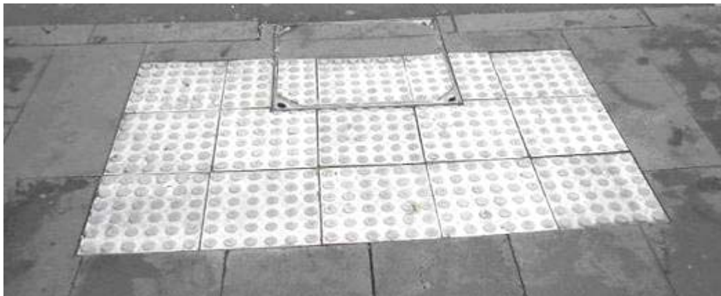
Photo 21: An example of how warning TSGI can be integrated into the design of utility service cover.
