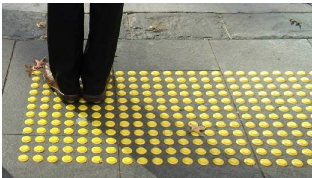
Photo 5: View of warning indicators. Note how the domes have been located to maintain equal spacing between domes across the entire warning indicator surface.
