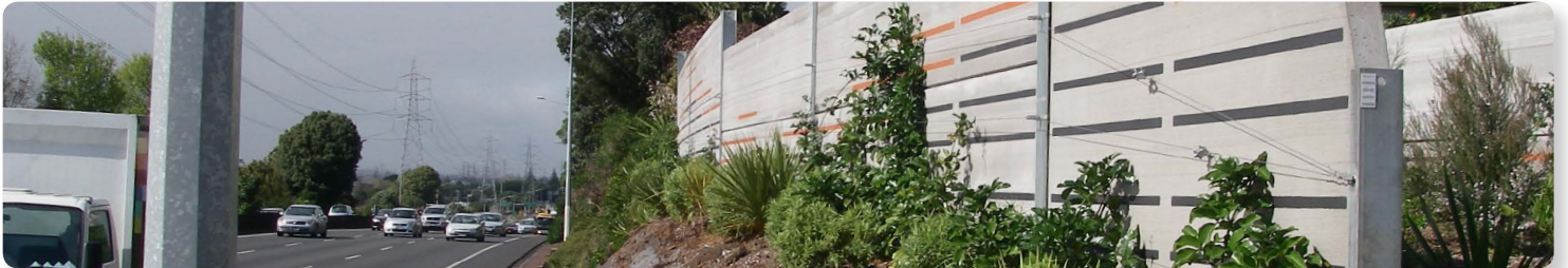
Noise barriers installed under the Noise Improvement Programme by the AMA at Otahuhu
