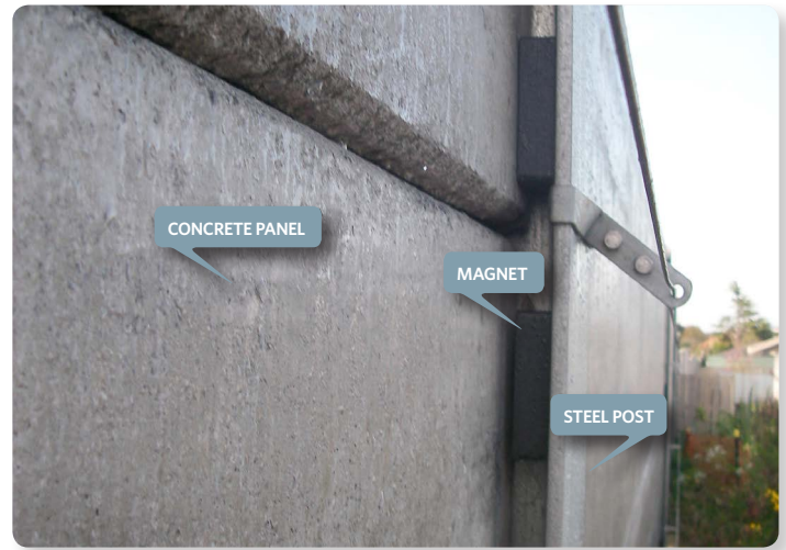
Ferrite magnets were used to pack gaps between noise barrier posts and panels
