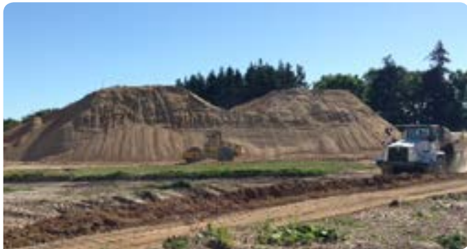
This huge pile of soil at the corner of Pickering Road and SH1 is 'preload' which has been put in place to consolidate the ground ahead of foundation works on the Pickering Road bridge. It will be in place for a couple of months, then will be removed in part to enable the construction of the bridge abutments.
