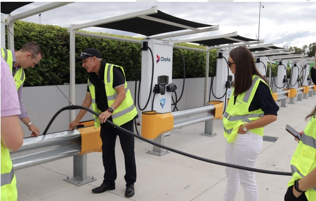
Figure 7: A support structure for the charging cable (Credit Meaghan Scanlon/LinkedIn)
