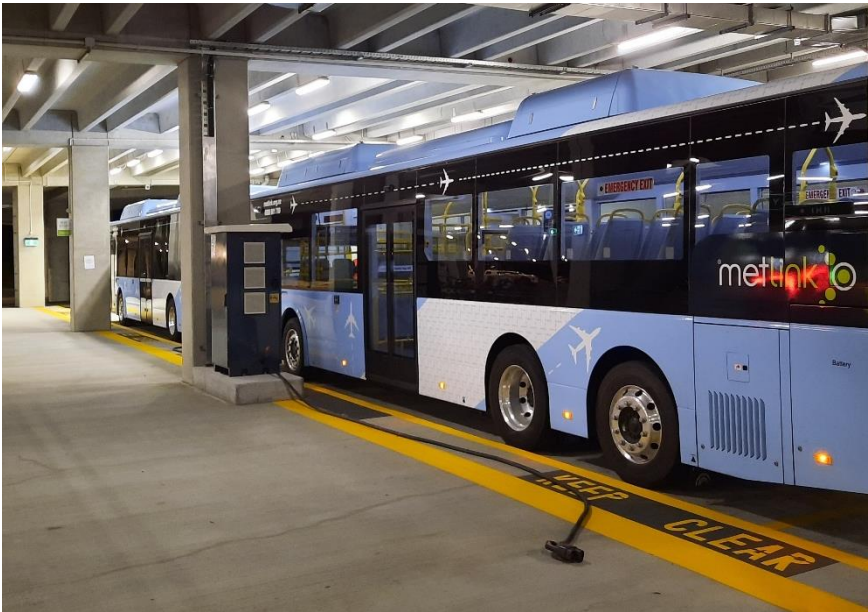
Figure 6: Wellington Airport have established capacity to charge two buses at a time by positioning a pedestal charger between two bus parking spaces and providing two relatively long cords (credit: Edward Wright)
