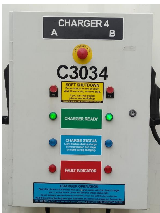
Figure 40: Wall mounted connection with an emergency stop button (Credit: Kirsten Boardman)
