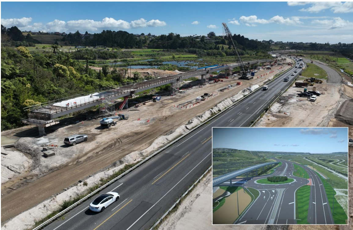
SH29 Takitimu Drive Toll Road and the new Takitimu Drive interchange under construction (looking towards Tauranga/Mount Maunganui)
