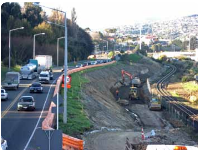
Site preparation work on the building of a 300 metre long retaining wall near the main truck railway line north of Barnes Drive
