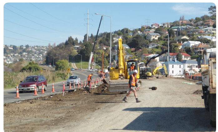
Earthworks and new storm water reticulation on both sides of the new Glen Bridge
