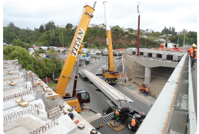
Work on preparing the placement of one of the beams on the new Glen Bridge
