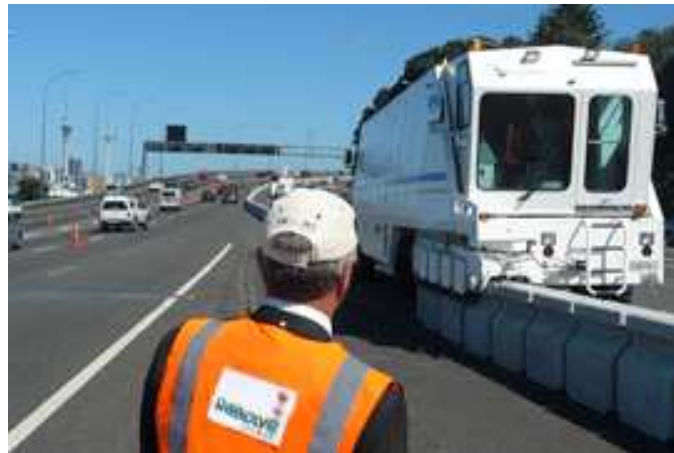
Lane Control with movable barrier - Auckland Harbour Bridge
