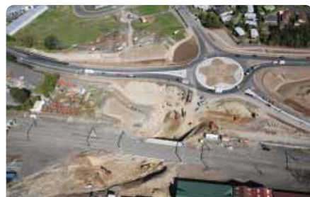
RIFLE RANGE ROAD ROUNDABOUT. An aerial view of the new Rifle Range Roundabout taken late August 2008, showing excavation almost completed for Norton Road
