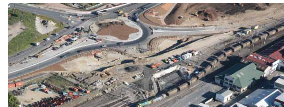
RIFLE RANGE ROAD ROUNDABOUT & NORTON ROAD RAIL BRIDGE CONSTRUCTION. This photo, taken on 28 May 2008, shows the Rifle Range Road Roundabout and the Norton Road rail bridge under construction. The complex construction sequence for the roundabout and rail bridge involved extensive collaboration between NZTA and ONTRACK and included the temporary relocation of Lincoln Street, the lowering of the entire Rifle Range Road Roundabout area by over three metres, the temporary diversion of two railway tracks, construction of a new rail bridge and the lowering of Norton Road by over seven metres to pass under the rail bridge.
