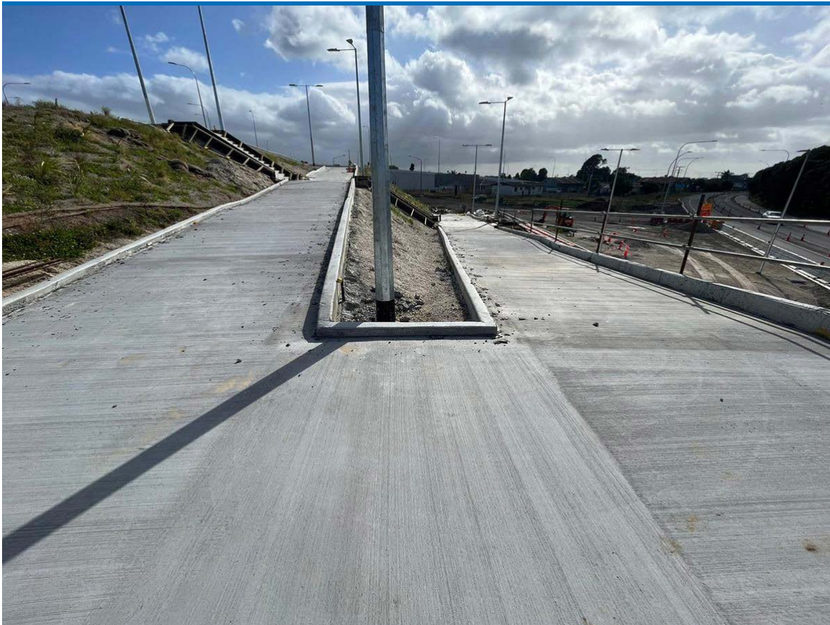
The new walking and cycling ramp connecting Te Maunga interchange and Truman Lane
