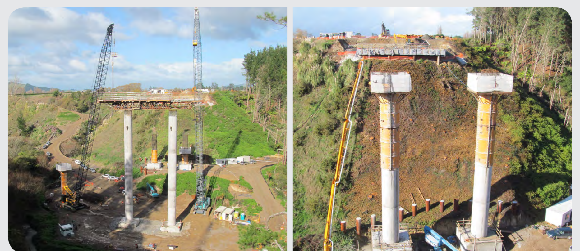
The viaduct columns are 2.6m diameter solid concrete. The two columns for the central pier are the tallest at a staggering height of 35m.
