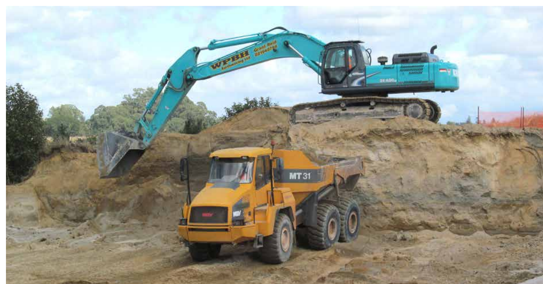
This is a 50 tonne excavator and a 30 tonne articulated dump truck working together on an excavation
