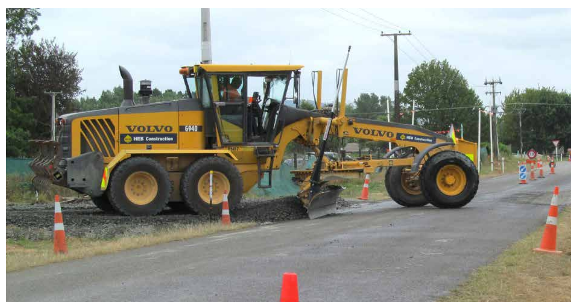
This grader is used to create a wide, flat surface before a road is sealed
