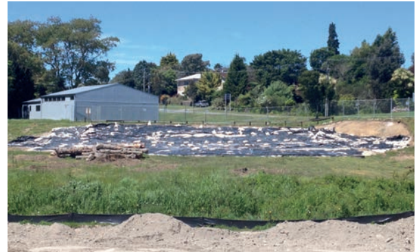
Asbestos site near Baden Powell Centre
