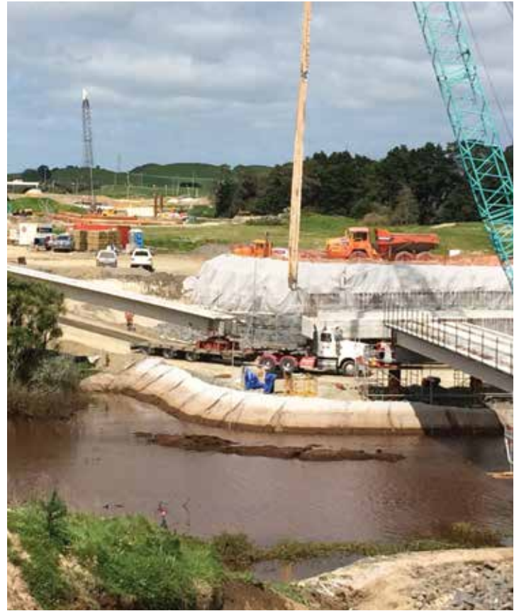
The beams were put in place on the Komakorau Stream bring during October.
