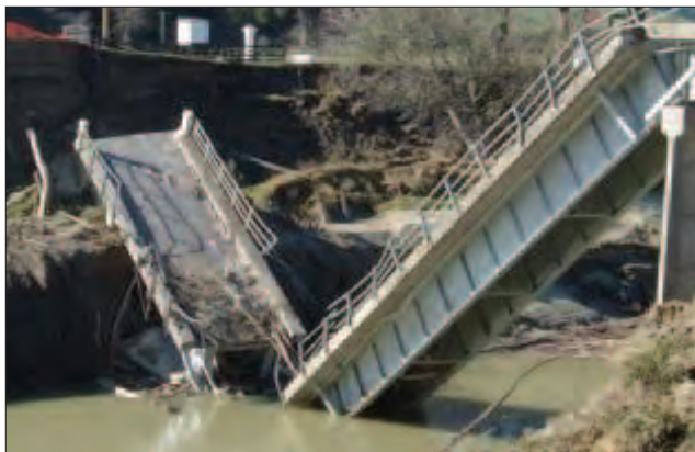
Flood-damaged bridge, Wanganui
