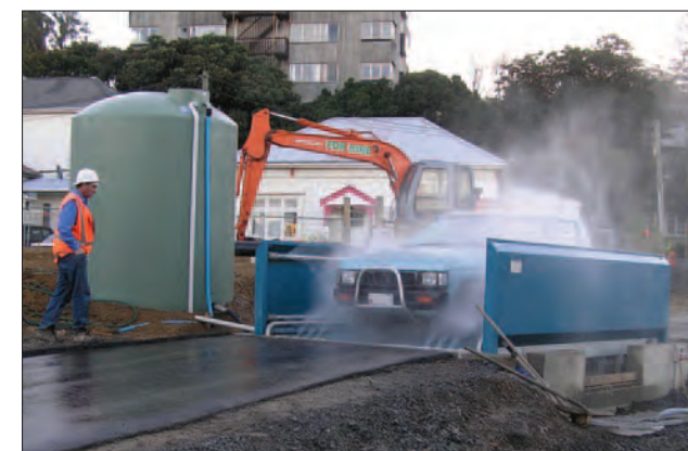
Wheel wash facility used to control dust from the Wellington inner city bypass project
