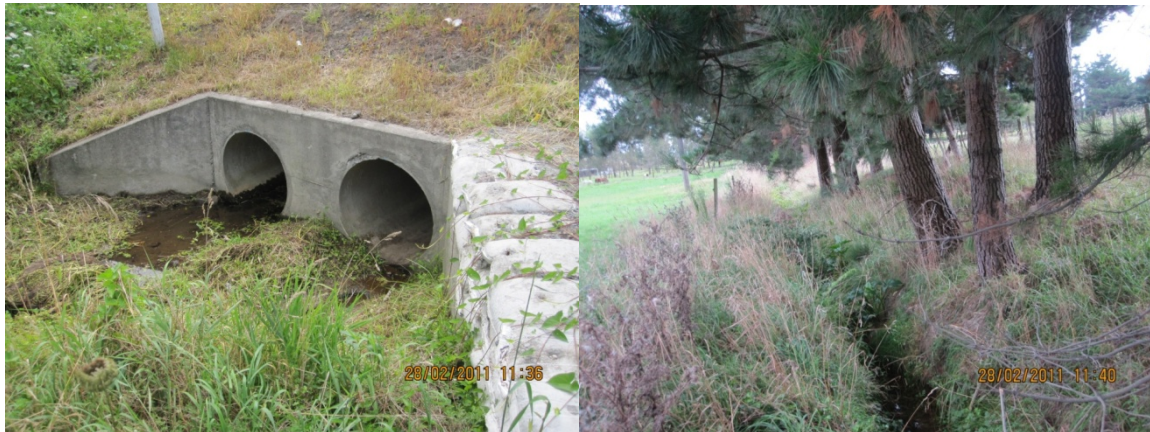
Photos 52 and 53: Hadfield/Te Kowhai Stream downstream, showing the SH1 culvert outlet (left) and a typical section of the stream (right).
