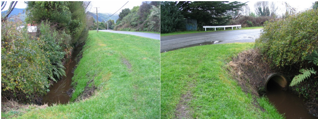
Photo 5 and 6: Drain 7 north, looking upstream of Rata Road (left) and to the culvert under Rata Road (right).
