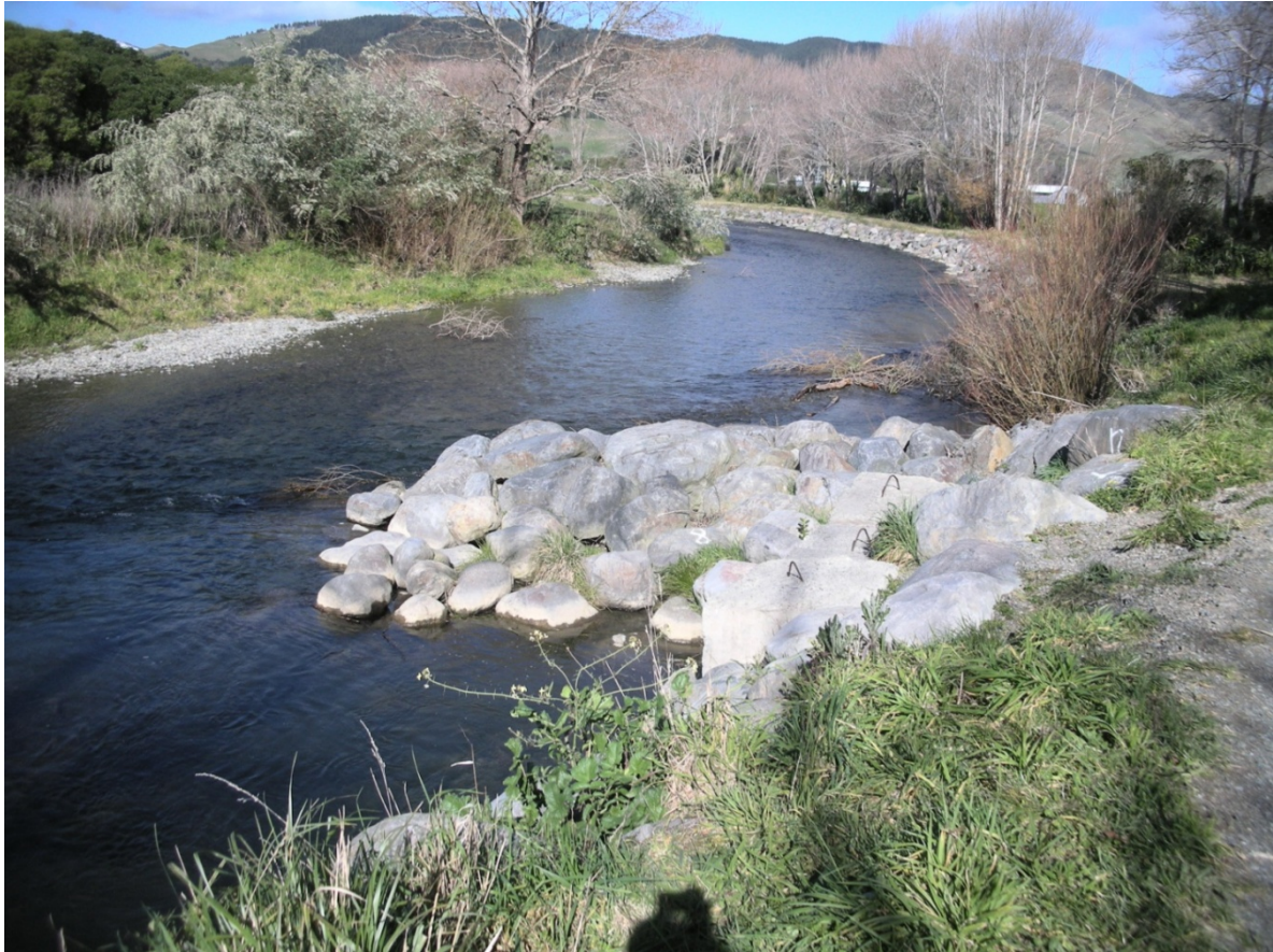
Photo 26: A GWRC construction groyne in the Waikanae River upstream of the proposed Expressway crossing. Rock armour to the bank can be seen in the background.
