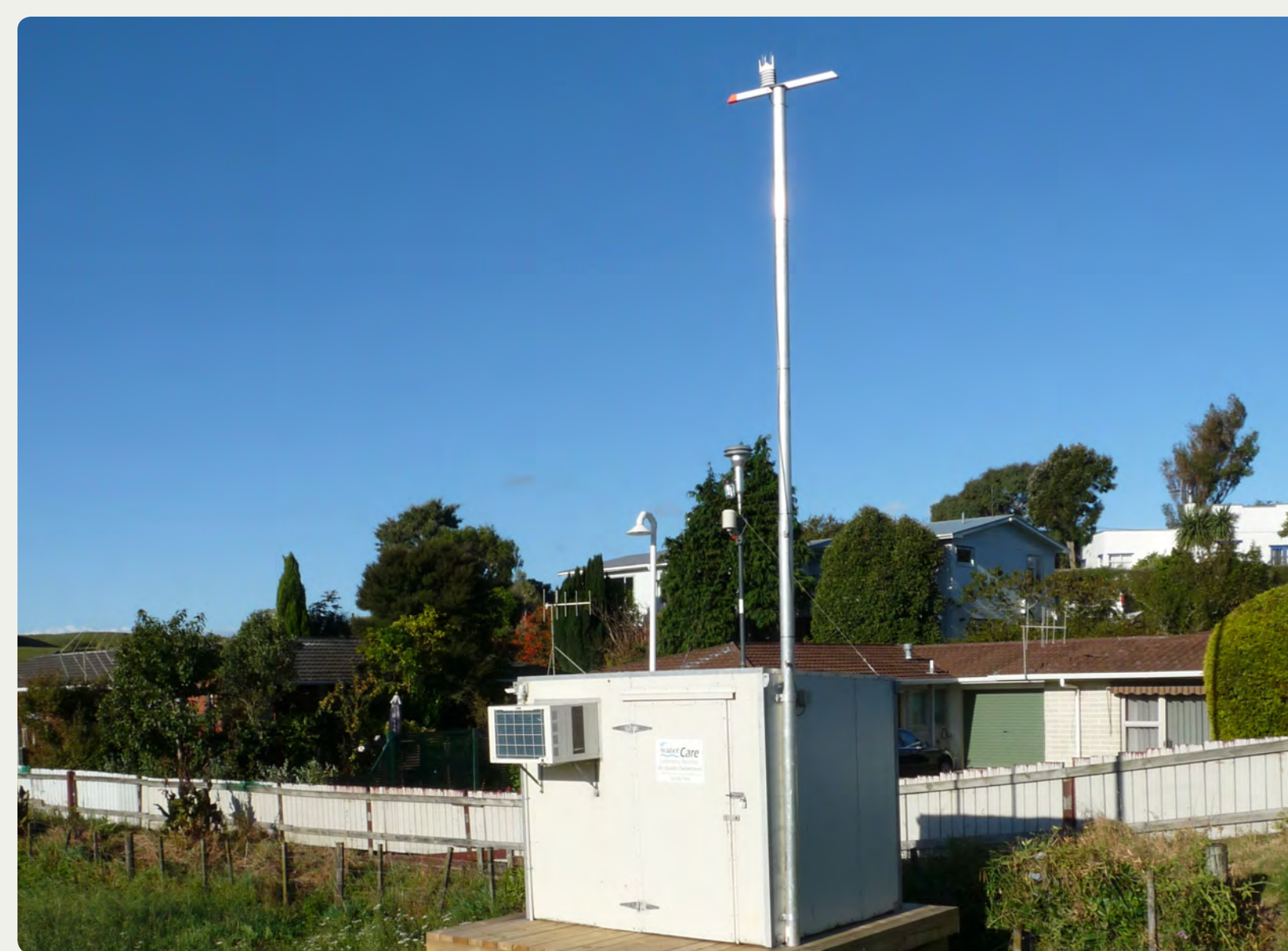
Air quality monitoring station on Raumati Road
