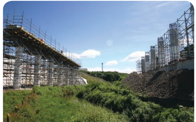
Constructing a bridge across the Puhinui Stream requires high standards of environmental management.
