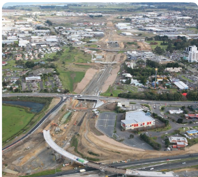
Pictured: Beam installation over SH1 and the view over the new motorway towards the West.
