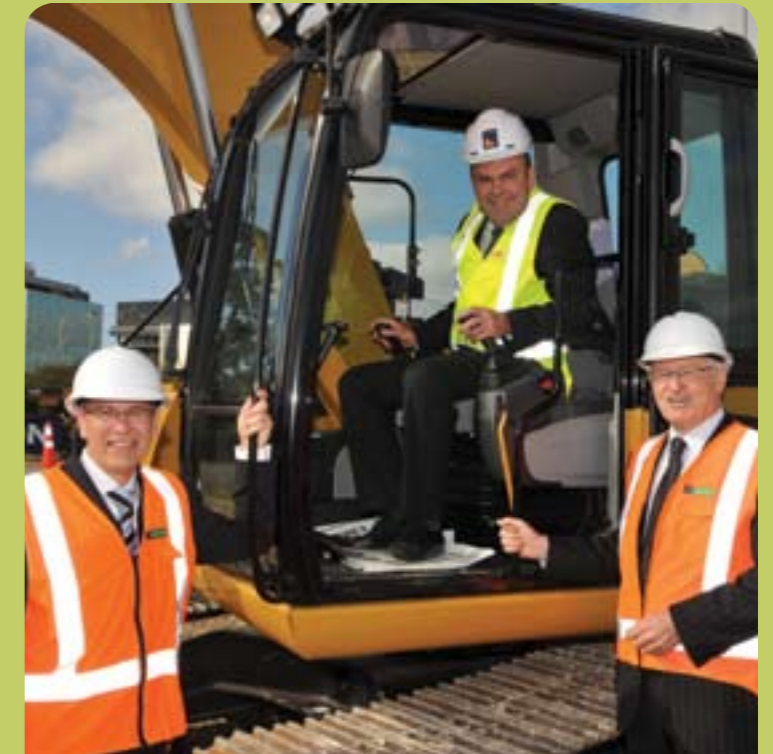
Minister of Transport Hon Steven Joyce starts construction of the Manukau Rail Station, alongside Kiwirail Chairman Jim Bolger and Manukau Mayor Len Brown.
