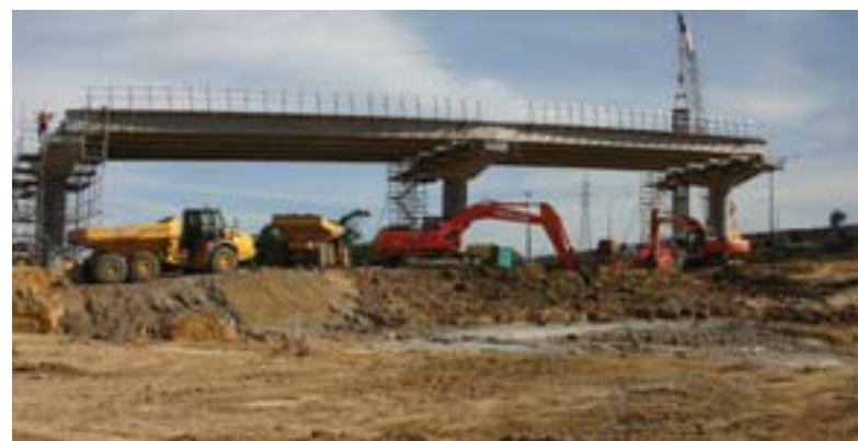
The piers and beams for the SH1-SH20 southbound link flyover are a new landmark for Manukau.
