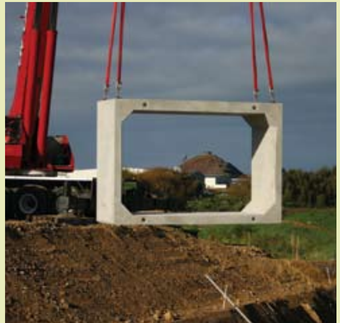
McLaughlin's Hill framed by a concrete culvert section being lifted into place.
