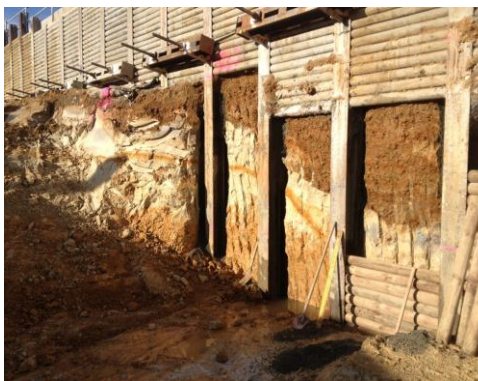
Soil strata in the area between HMNZS Olphert and the War Memorial at the Taranaki Street end of the site; the trench is about 6m deep at this point
