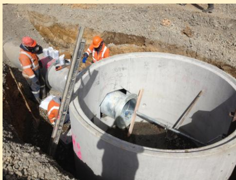
Manhole chamber at Cambridge Terrace. A valve is being installed in the manhole which is why it is so big.
