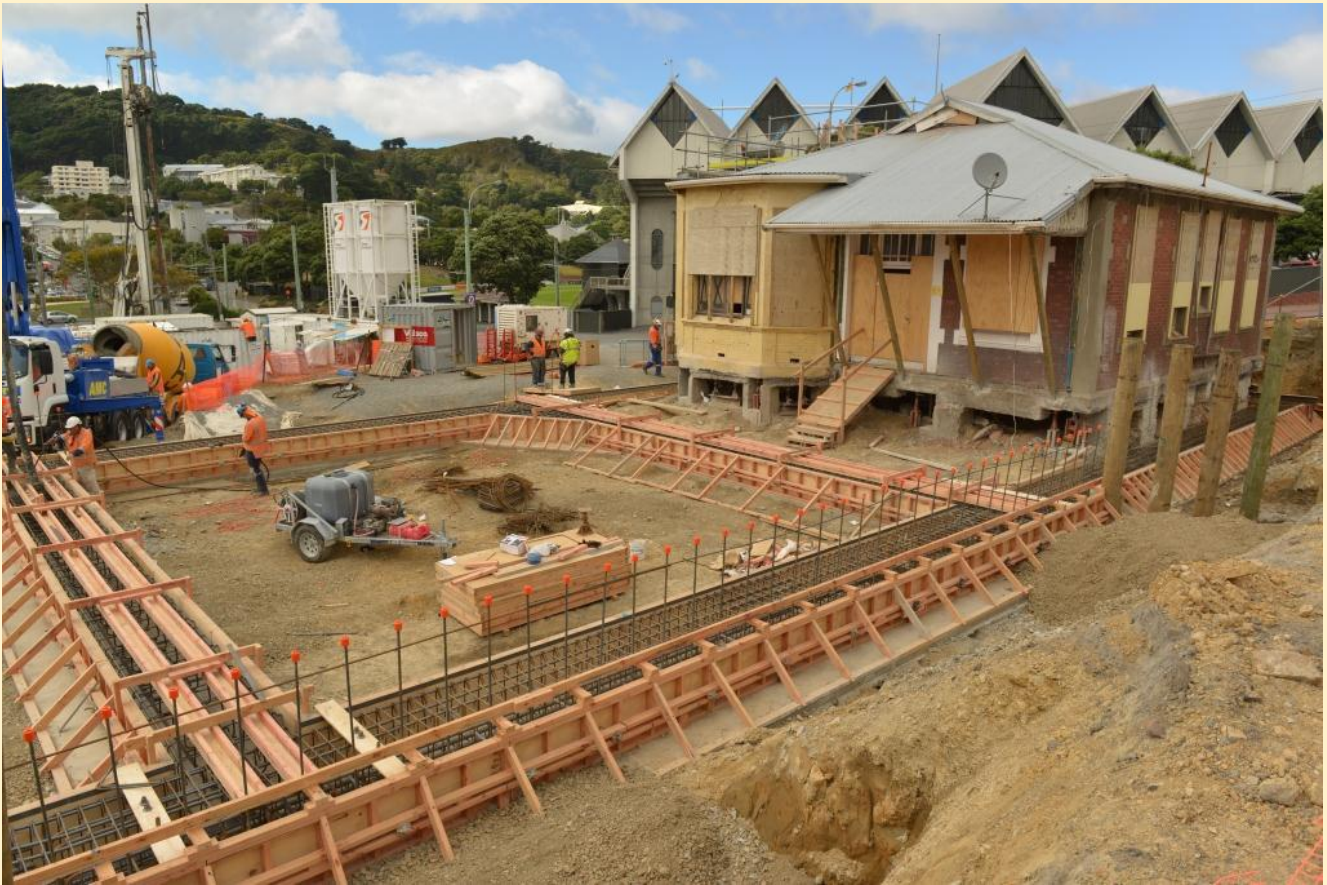
13 March 2014: The stripped-down and strengthened Home of Compassion Crèche awaits construction of the rail system to move it back into the site, the first of three moves to relocate it within the Memorial Park.
