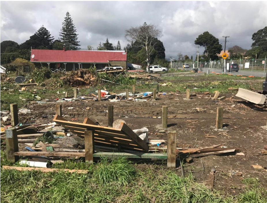
Vacant residential building and stockpiled remains of previously demolished buildings, taken from the western corner, facing south east (photo taken: September 2017)
