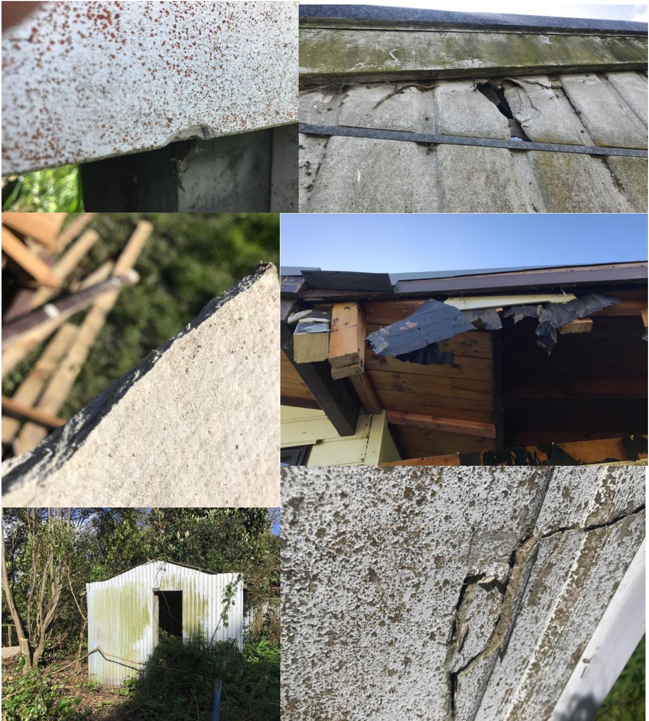
The buildings are constructed of wood, brick, metal, corrugated plastic, aluminium composite material and fibrolite with concrete slabbing (photos taken: September 2017)
