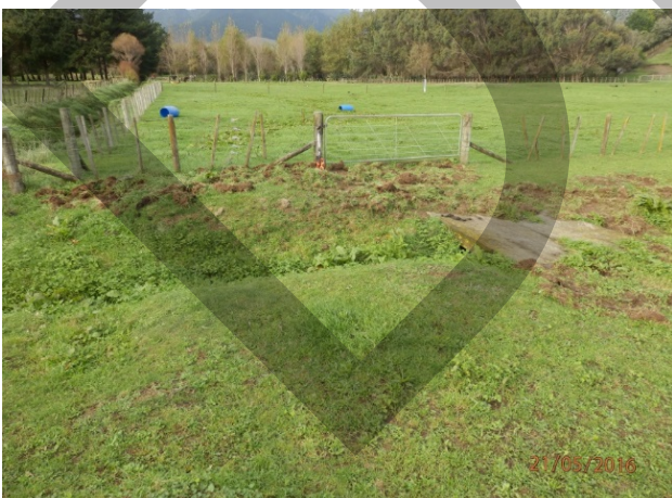
Fig. 3 Central bridge and drain: to be railed as an maintenance access point.
