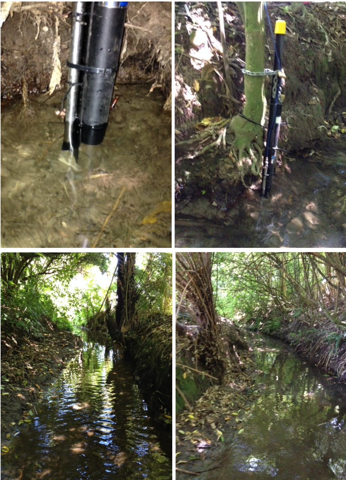
Figure 2.4: Water level and turbidity sensor installation on the Mangapouri Stream.
