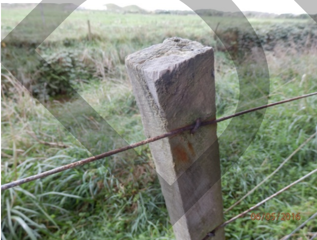
Fig. 3 Corroded wire and staple.
