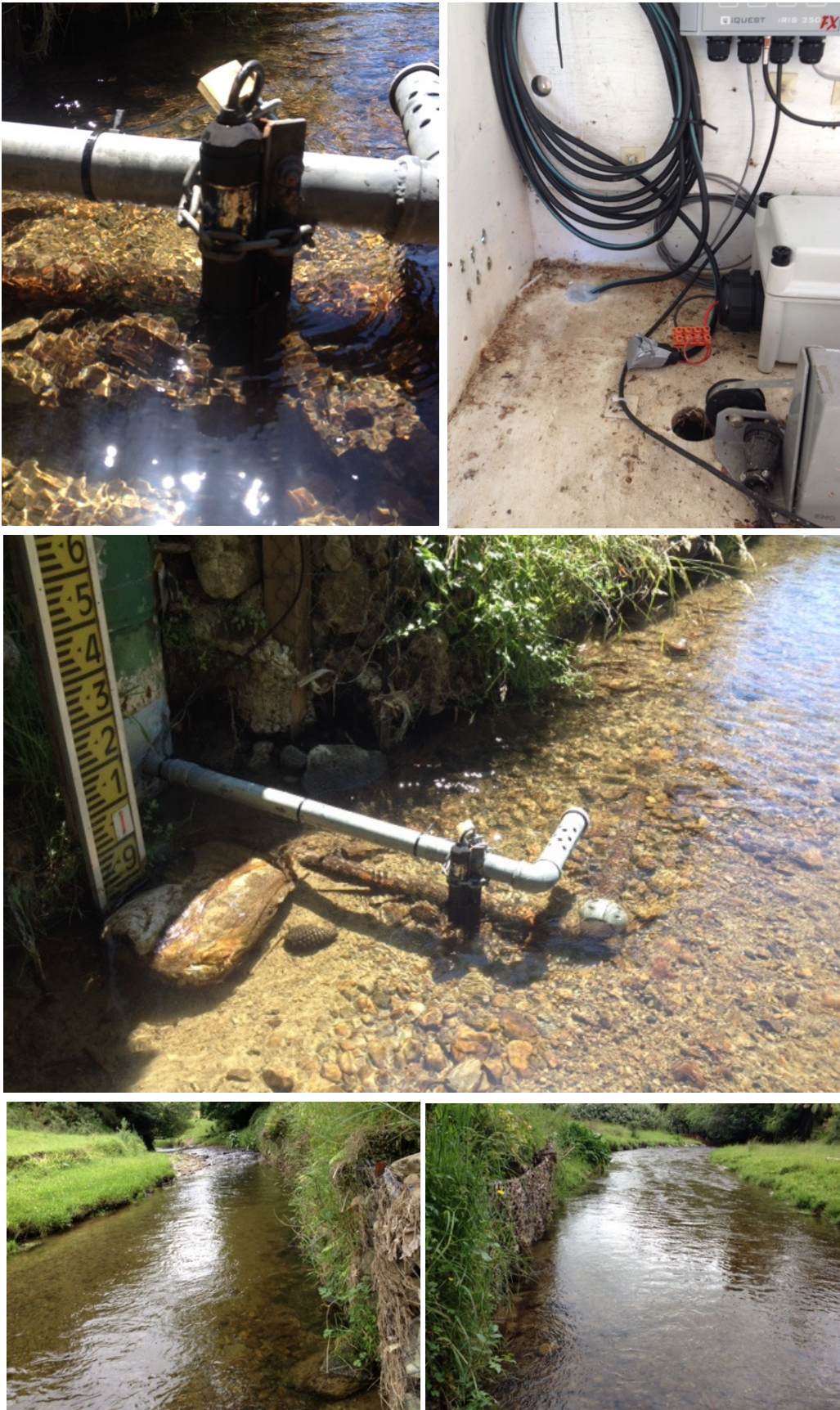
Figure 2.3: Sensor installation on the Mangaone Stream at Ratanui.
