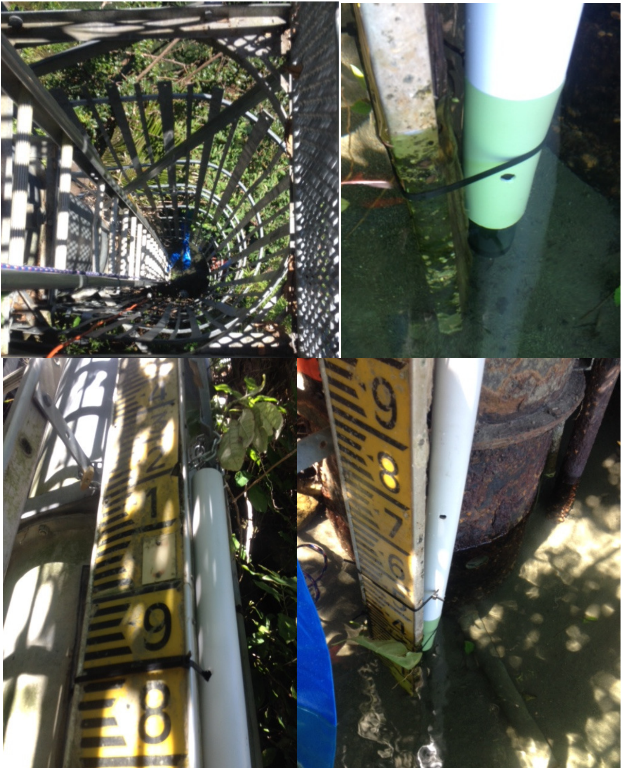
Figure 2.2: Sensor installation on the Otaki River at Pukehinau.
