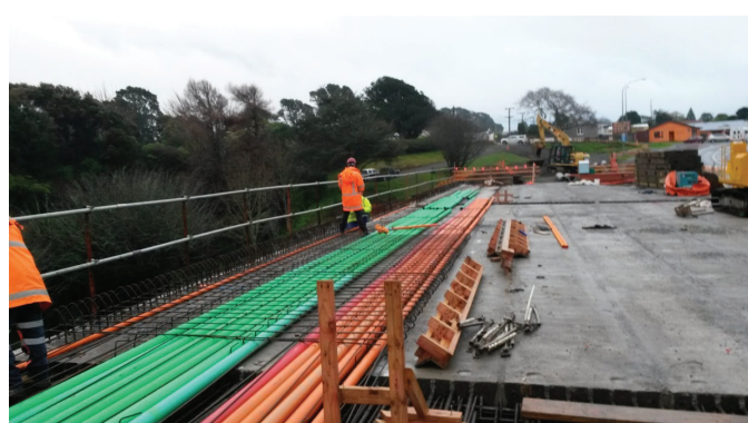
Service ducts being installed under the footpath on the new Te Henui Bridge.
