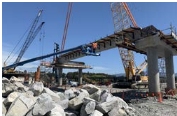
A major milestone - the first of the 52 tonne 'super tee' bridge beams being put in place.
