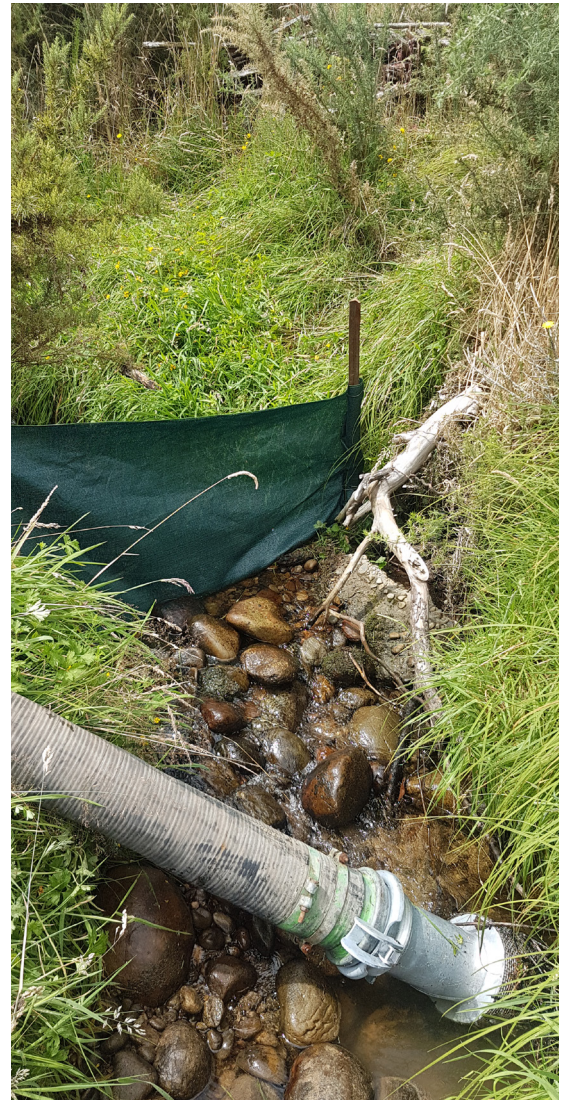
A screen protects fish while a pump redirects water from Ahaura Stream as part of ecology protection measures.
