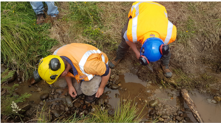
To protect Ahaura Stream from trucks and equipment coming on-site, a temporary culvert was put in place and the stream was diverted. Contractors helped to safely relocate fish from the stream.
