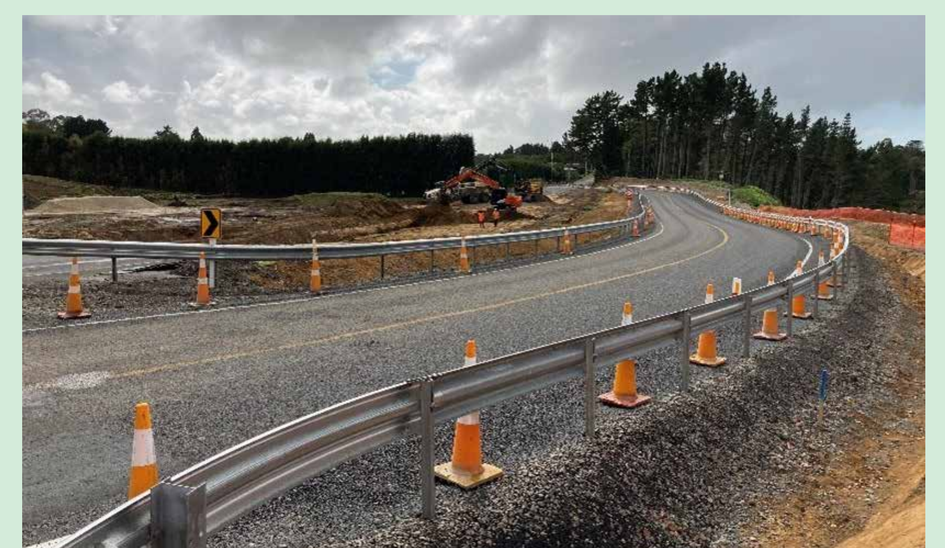
A diversion road has been completed and opened at Wairoa Road, ahead of construction starting mid-May for the Wairoa Road Overbridge.
