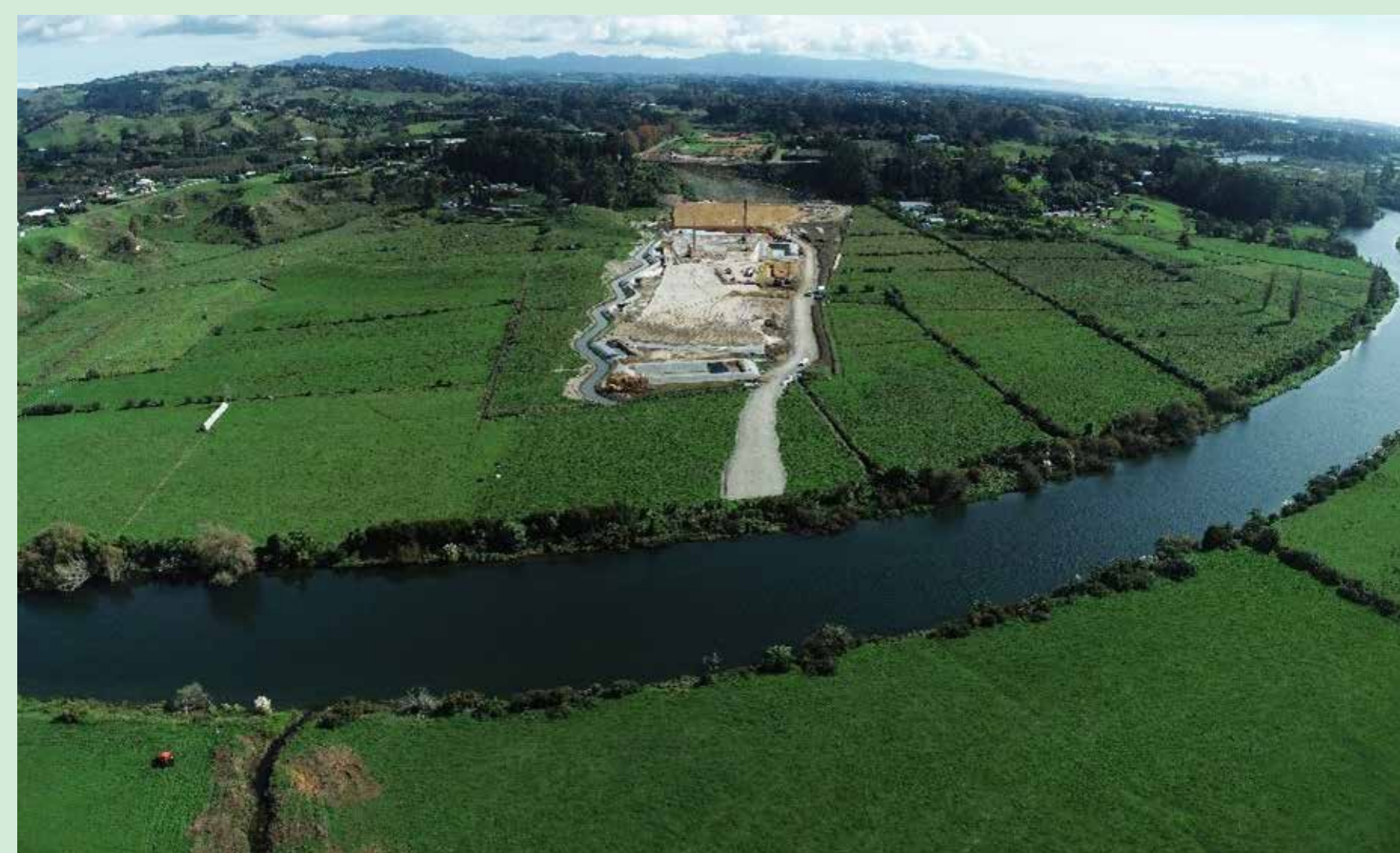
Aerial photo taken April 2022, looking towards Wairoa Road, and onward to Te Puna. Wairoa Awa (river) is in the foreground. Work starts on the Wairoa Awa staging bridge early June.
