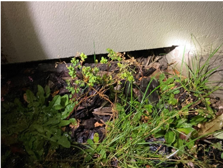
Figure 2 Typical picture of gap under noise wall
