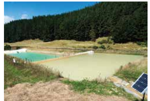
Above: Dirty water makes its way into the sediment-retention pond's first bay, where a coagulant is added to help settle sediment out of the water.
