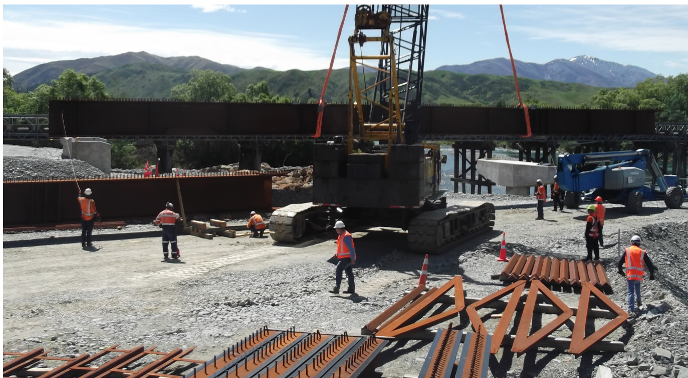
Beam placement at the No 2 bridge on the Kurow side of the river.
