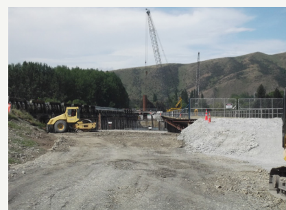
Road formation work on the new No 1 Bridge on the Hakateramea side of the river.
