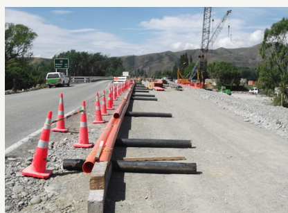
Duct installation preparation on the approaches to the new No 2 bridge near Kurow.
