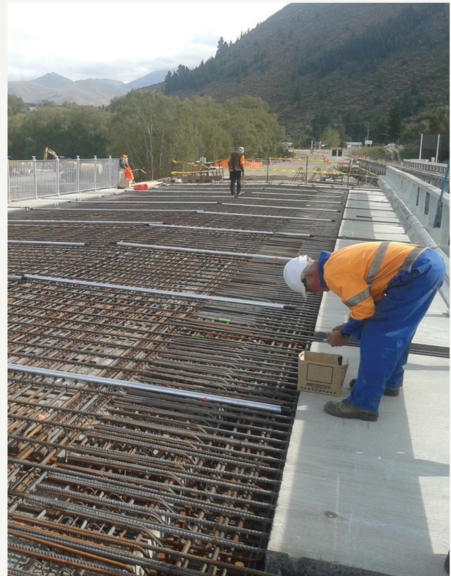
Bridge No. 2 steel work for the deck - view from the island to Kurow.
