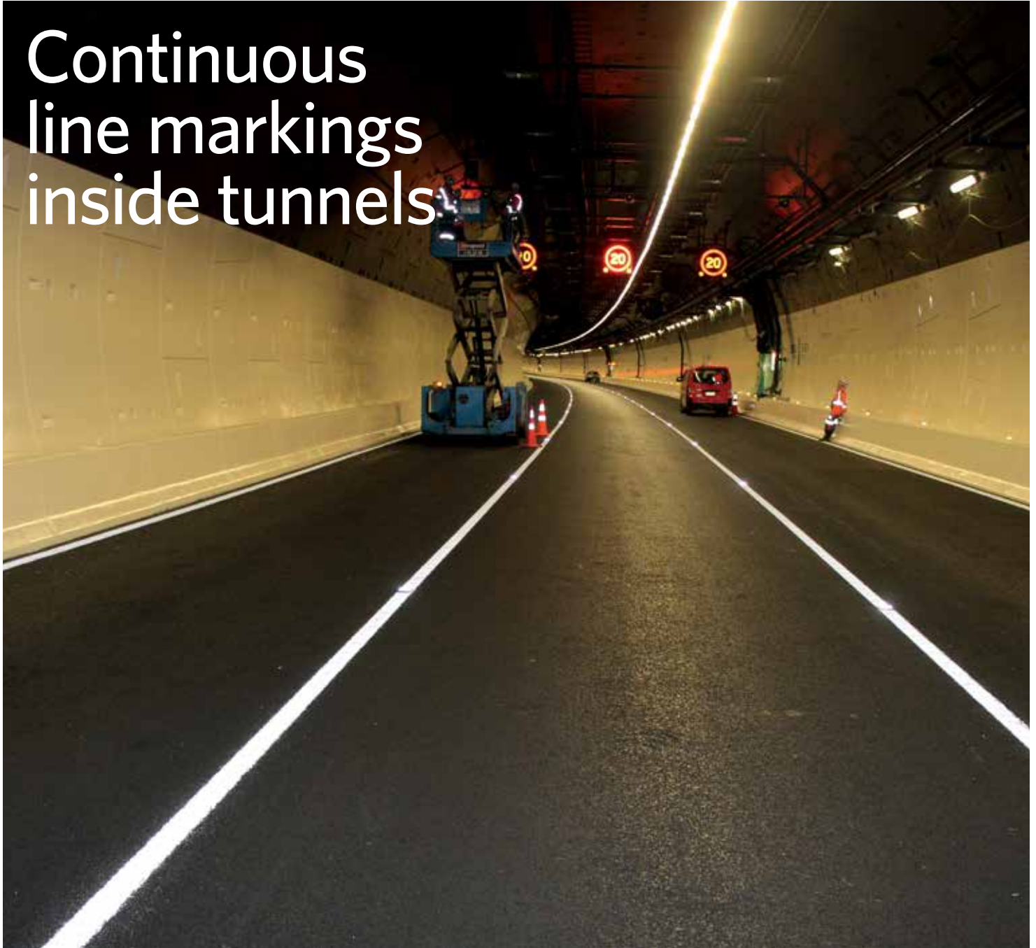
Continuous line markings will indicate to drivers to not change lanes inside both tunnels.
