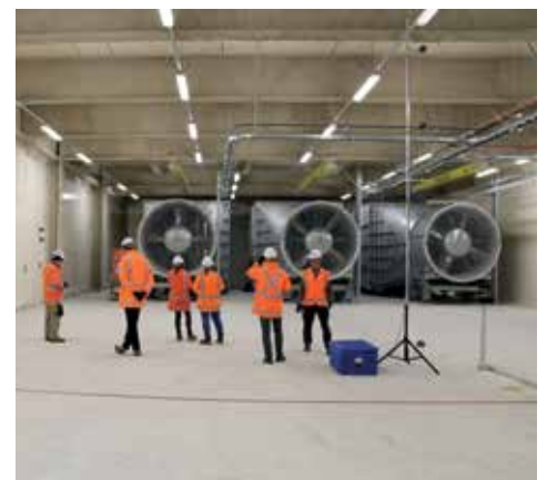
Anemometer grid air flow testing by the commissioning team.
