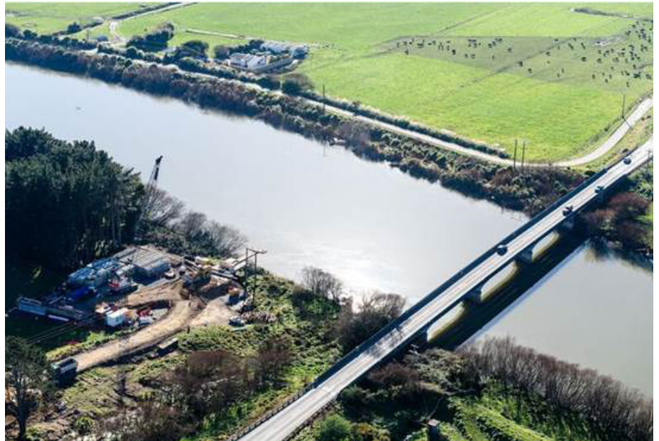
Aerial view of the Manawatū River Bridge and the early stages of temporary bridge construction
