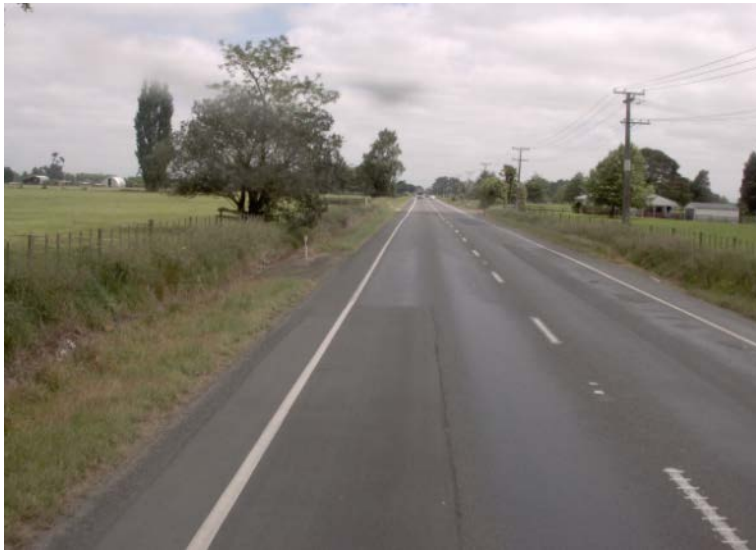
Figure C.38 Mill and AC patch - SH27-46-17455-17471 (decreasing side) - 16- month inspection
