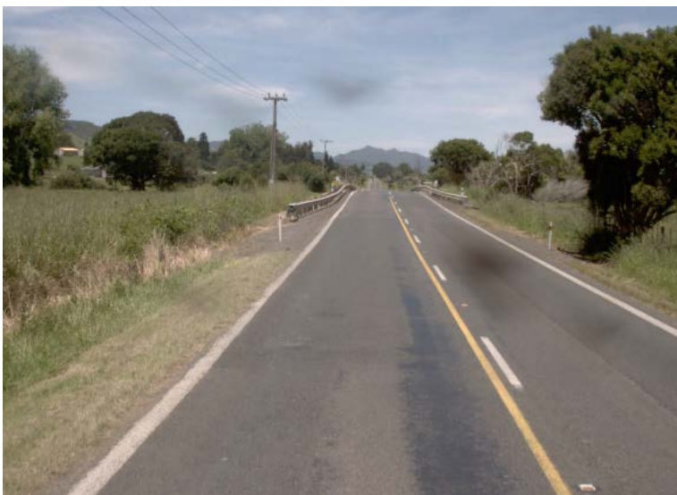
Figure C.15 3% in- situ stabilisation – SH26–S80–13577–13584 (decreasing side) – 16- month inspection
