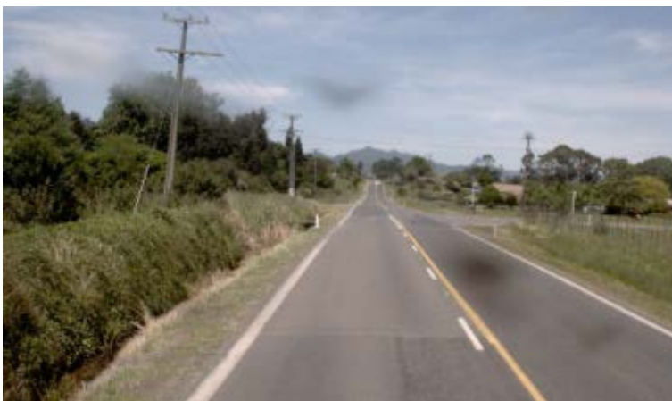
Figure C.23 Full depth granular reconstruction – SH26-RS80-13394-13434 (decreasing side) – 16- month inspection
