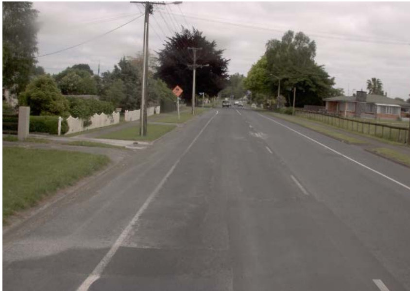
Figure C.6 1.5% in- situ stabilisation – SH24 –RS0 – 1465 – 1485 – 16- month inspection
