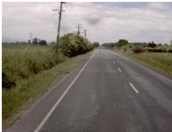
Figure 5.1 Rutting and cracking after 16 months in the SH27 full depth granular reconstruction site which was also stabilised with 1.5% cement
