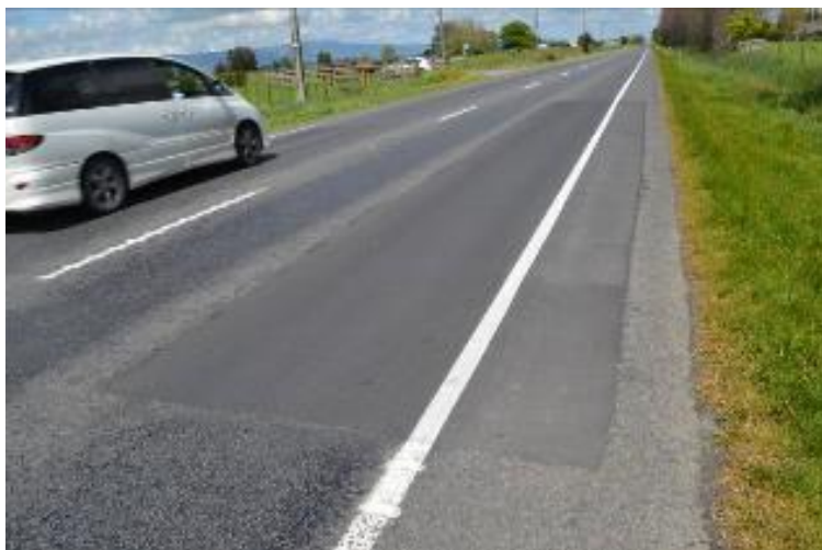
Figure C.37 Mill and AC inlay – SH27-46-17455-17471 (decreasing side) – 3- month inspection
