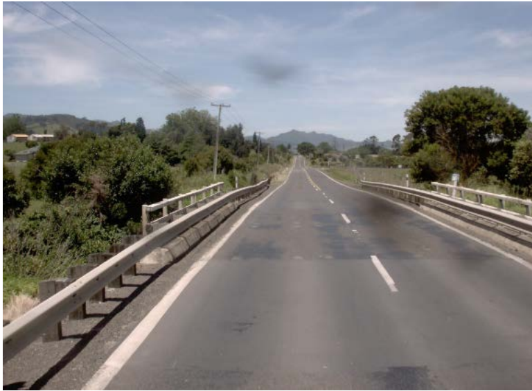
Figure C.26 Mill and AC patch - SH26-RS80-13596-13606 (decreasing side) - 16- month inspection
