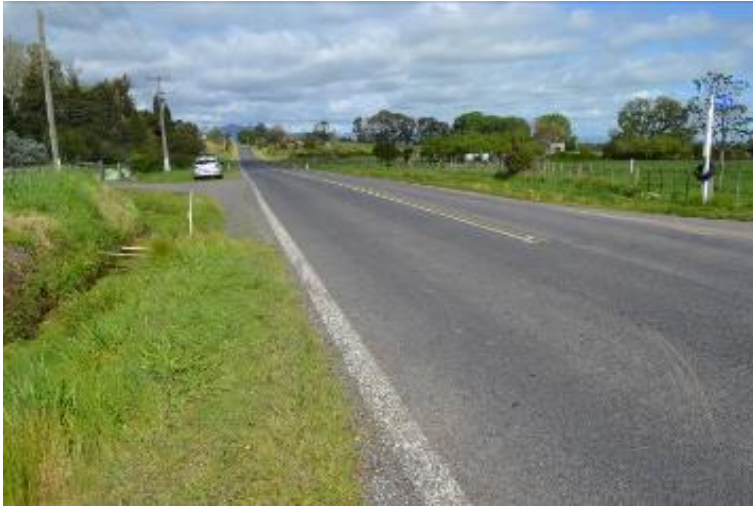
Figure C.22 Full depth granular reconstruction – SH26-RS80-13394-13434 (decreasing side) – 3- month inspection
