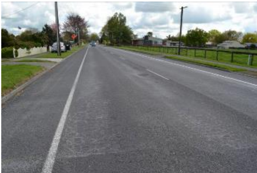
Figure C.5 1.5% in- situ stabilisation – SH24-RS0-1465-1485 – 3- month inspection
